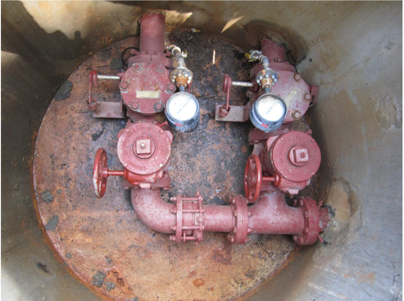
PHOTO 2: VALVE PIT PIPING AND PRESSURE GAUGES
