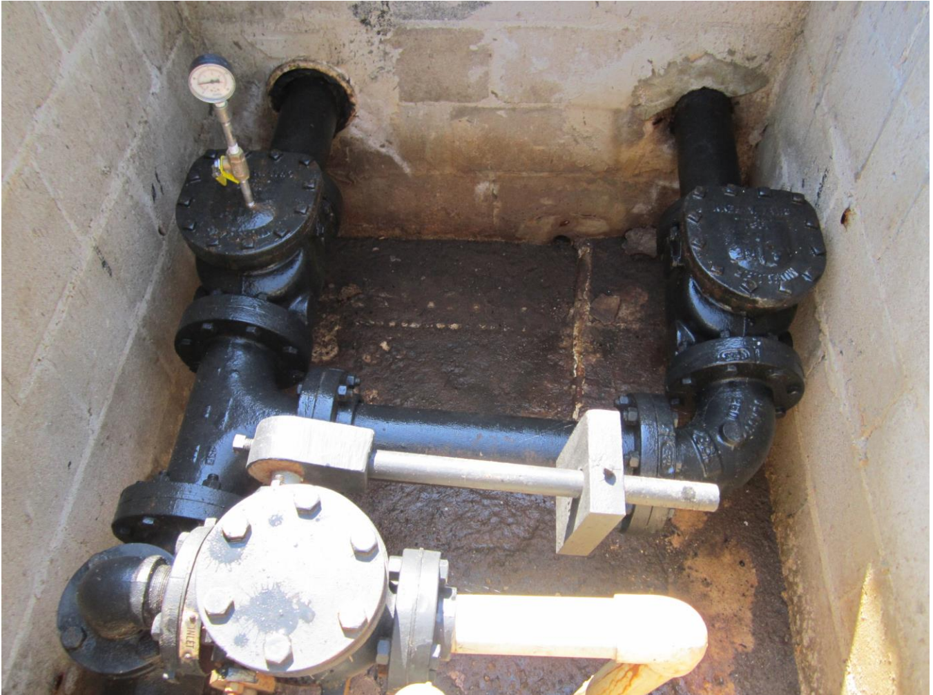
PHOTO 2: VALVE PIT PIPING AND PRESSURE GAUGE
