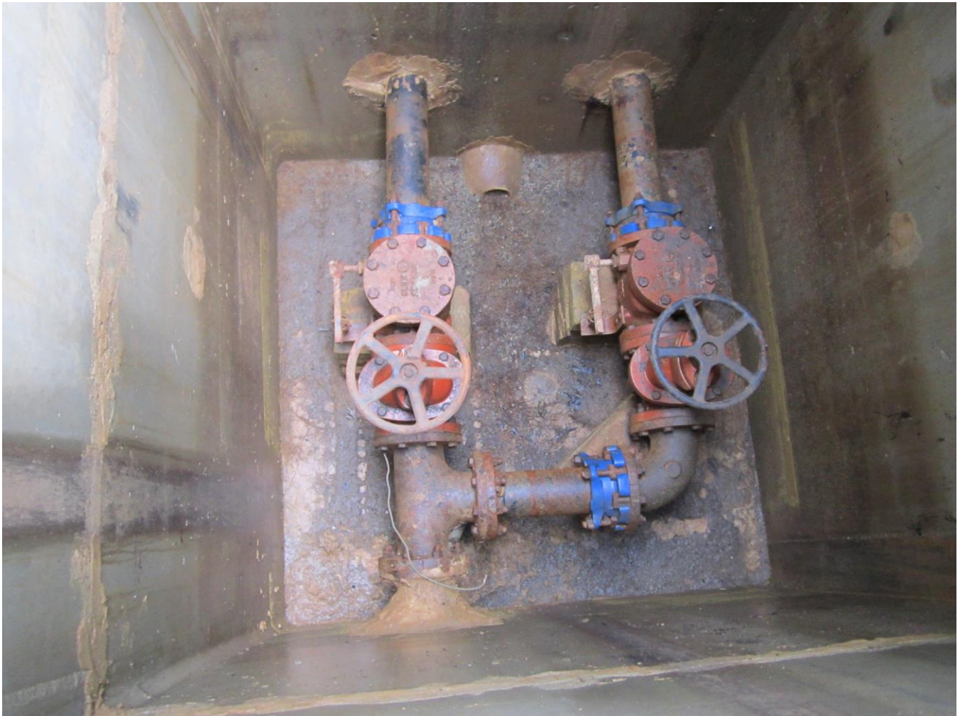
PHOTO 2: VALVE VAULT PIPING
