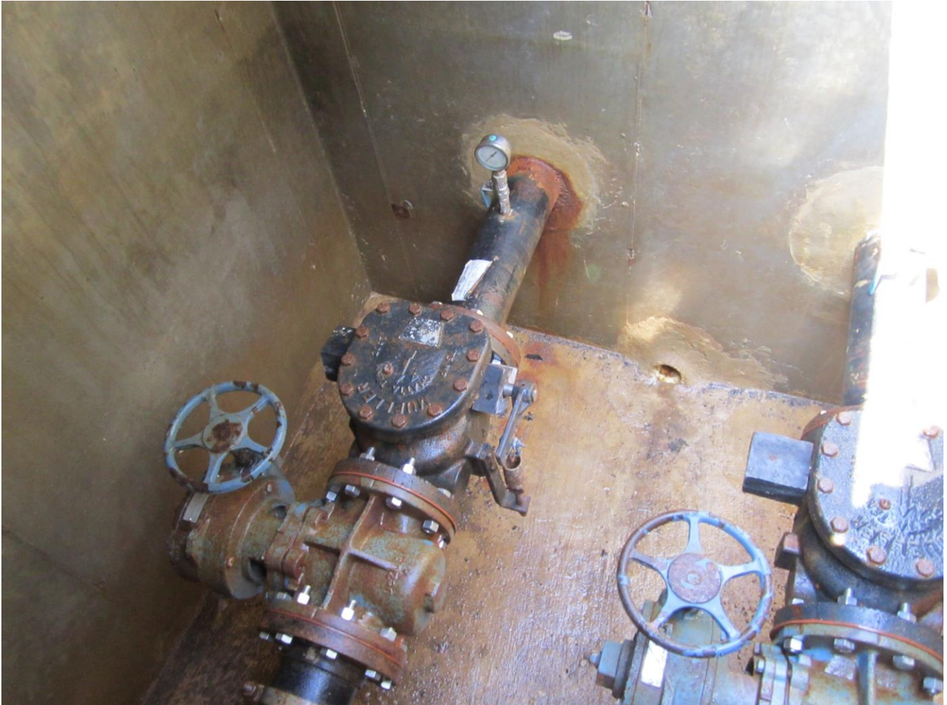
PHOTO 2: VALVE PIT PIPING AND PRESSURE GAUGE
