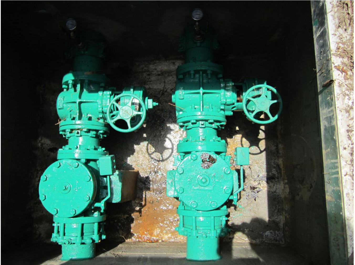
PHOTO 2: VALVE PIT PIPING AND PRESSURE GAUGES
