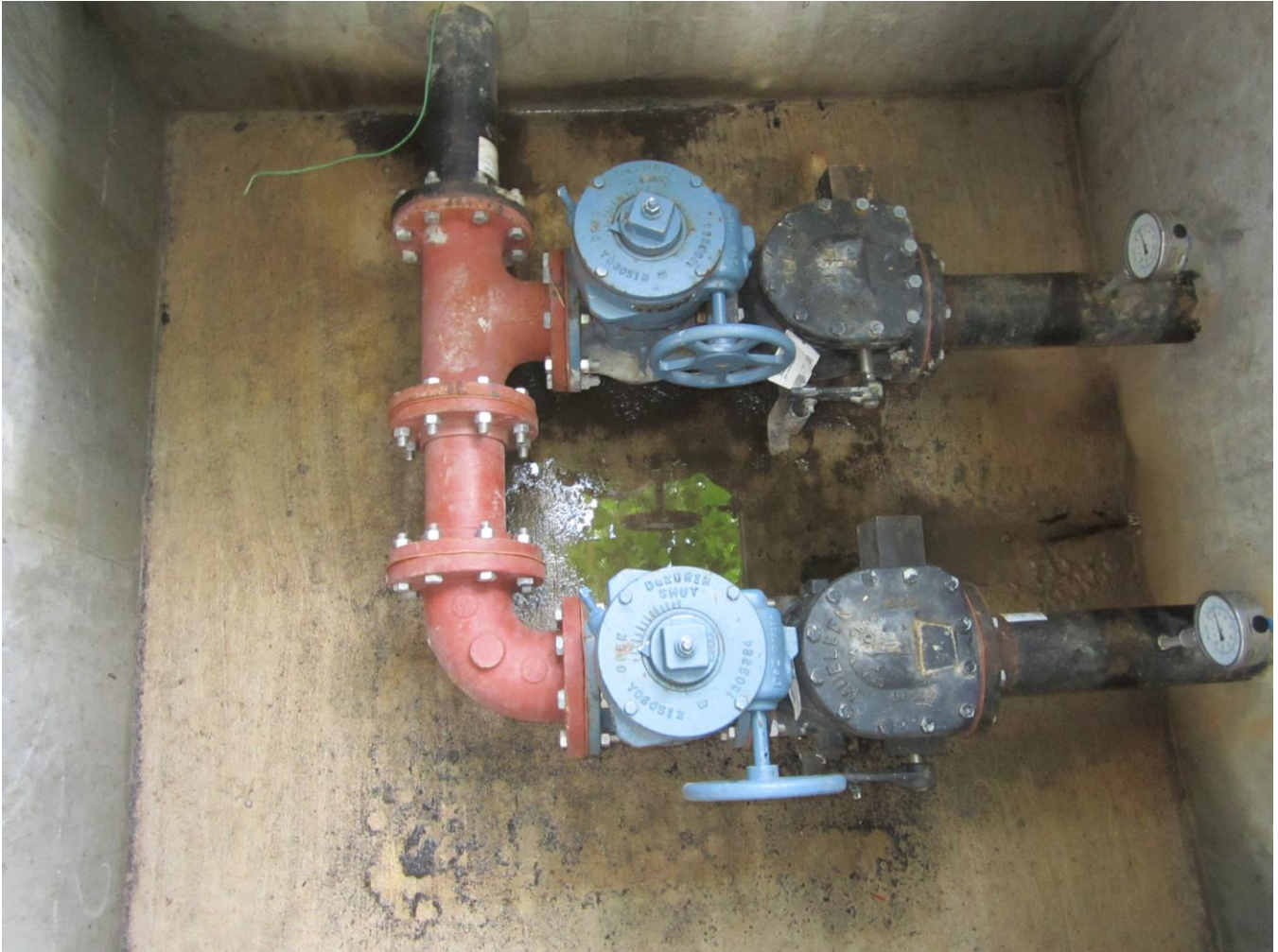
PHOTO 2: VALVE PIT PIPING AND PRESSURE GAUGES
