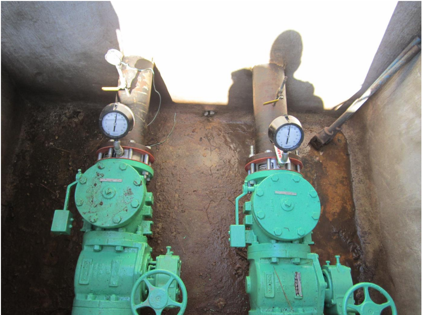
PHOTO 2: VALVE PIT PIPING AND PRESSURE GAUGES
