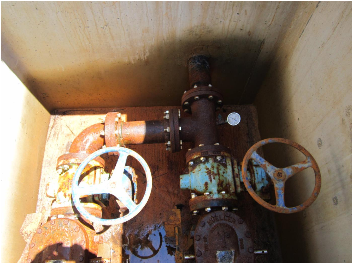
PHOTO 2: DISCHARGE HEADER PRESSURE GAUGE
