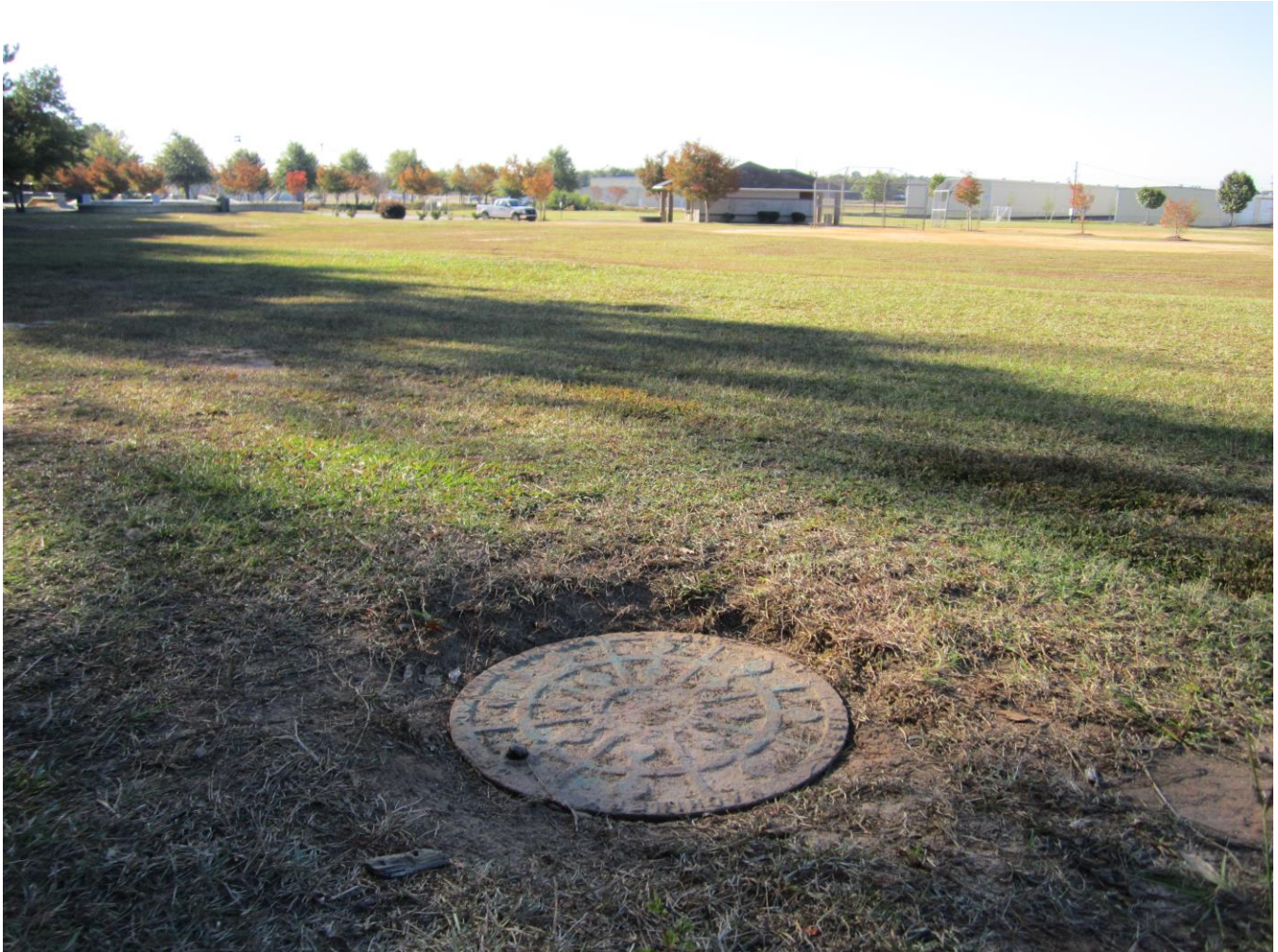
PHOTO 2: DISCHARGE MANHOLE AND PUMP STATION IN BACKGROUND
