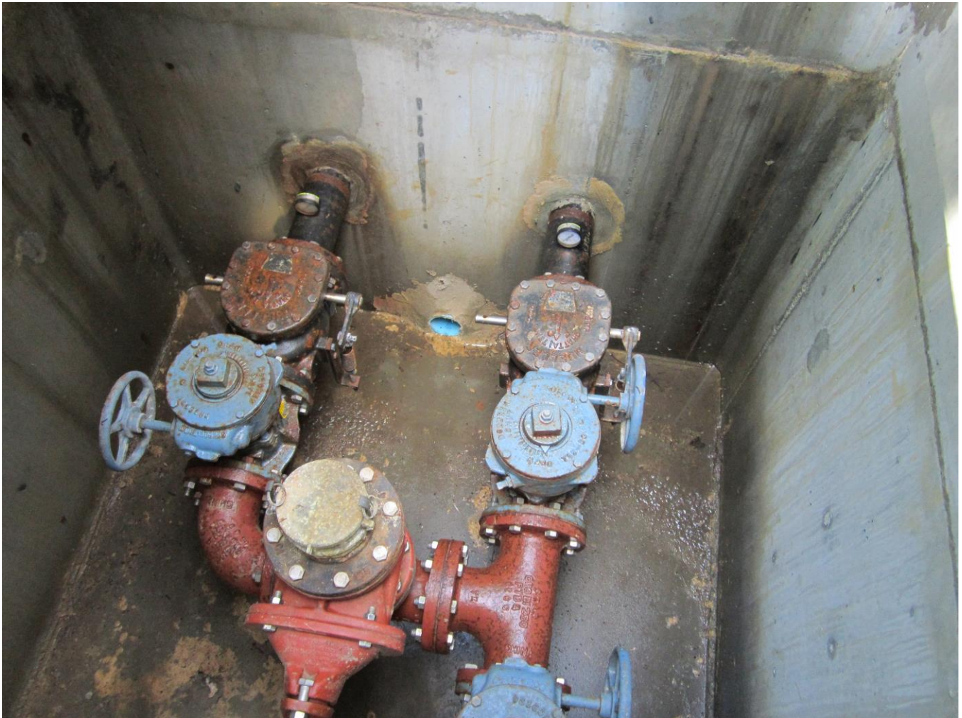
PHOTO 2: VALVE VAULT PIPING, BYPASS AND PRESSURE GAUGE
