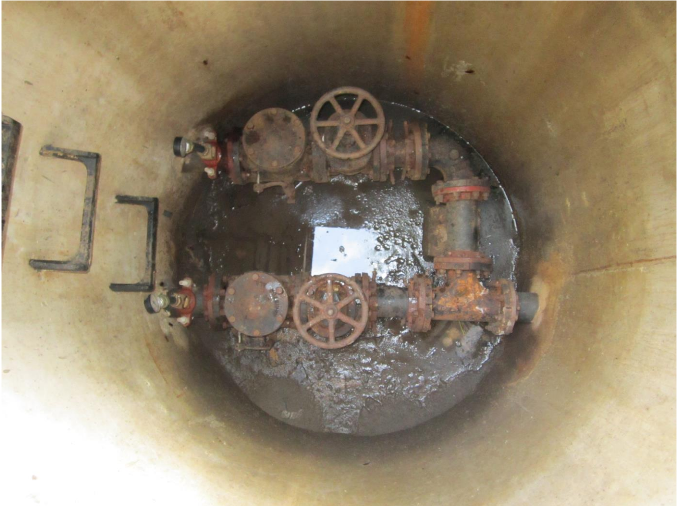
PHOTO 2: VALVE PIT PIPING AND PRESSURE GAUGES
