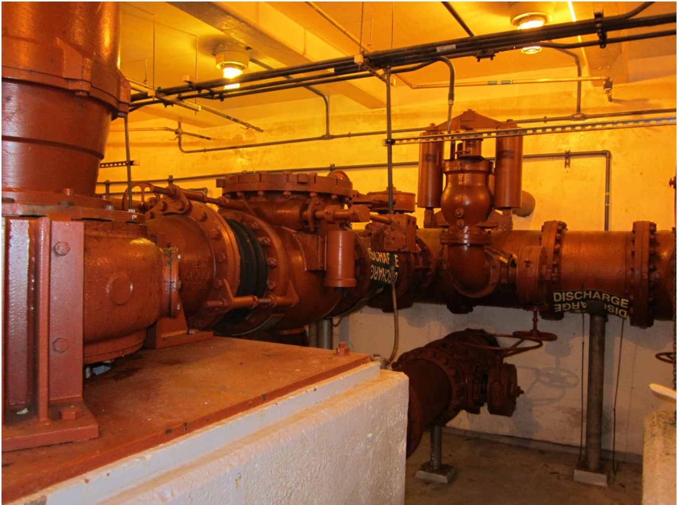
PHOTO 2: DISCHARGE HEADER PIPING
