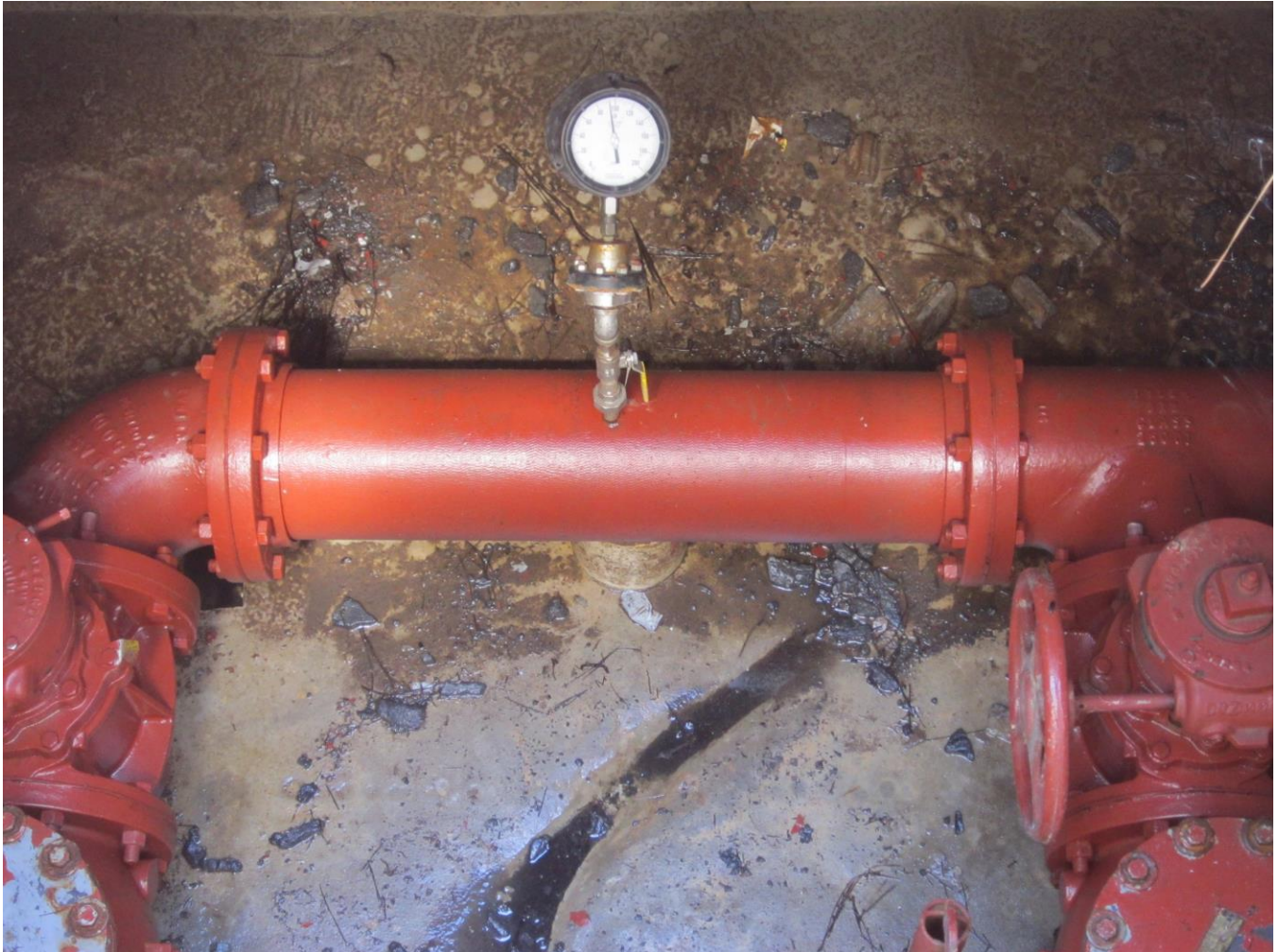
PHOTO 2: DISCHARGE HEADER PRESSURE GAUGE
