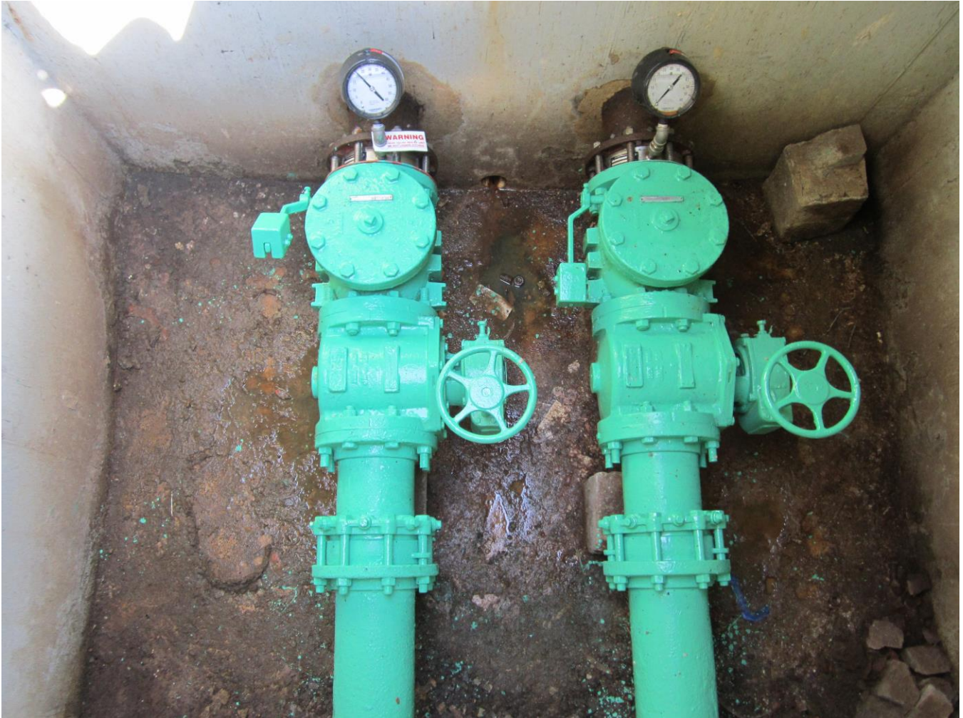
PHOTO 2: VALVE PIT PIPING AND PRESSURE GAUGES
