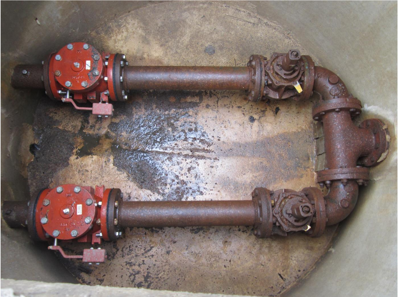
PHOTO 2: VALVE PIT PIPING
