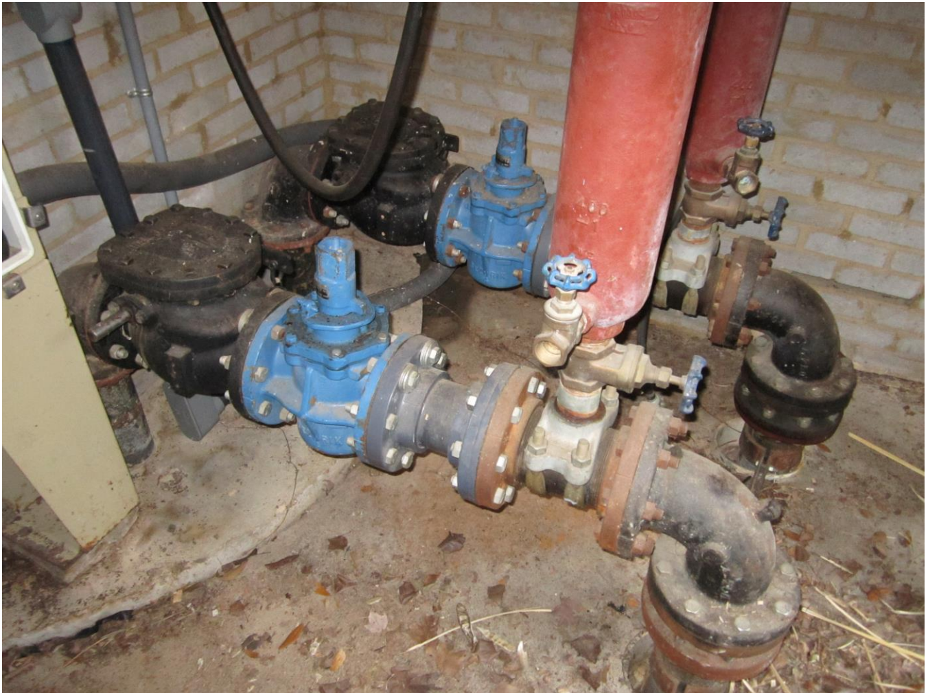
PHOTO 2: DISCHARGE PIPING HEADER
