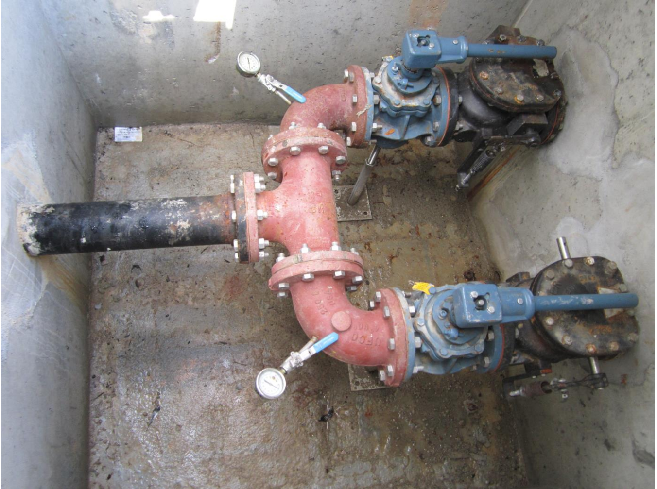
PHOTO 2: VALVE PIT PIPING AND PRESSURE GAUGES
