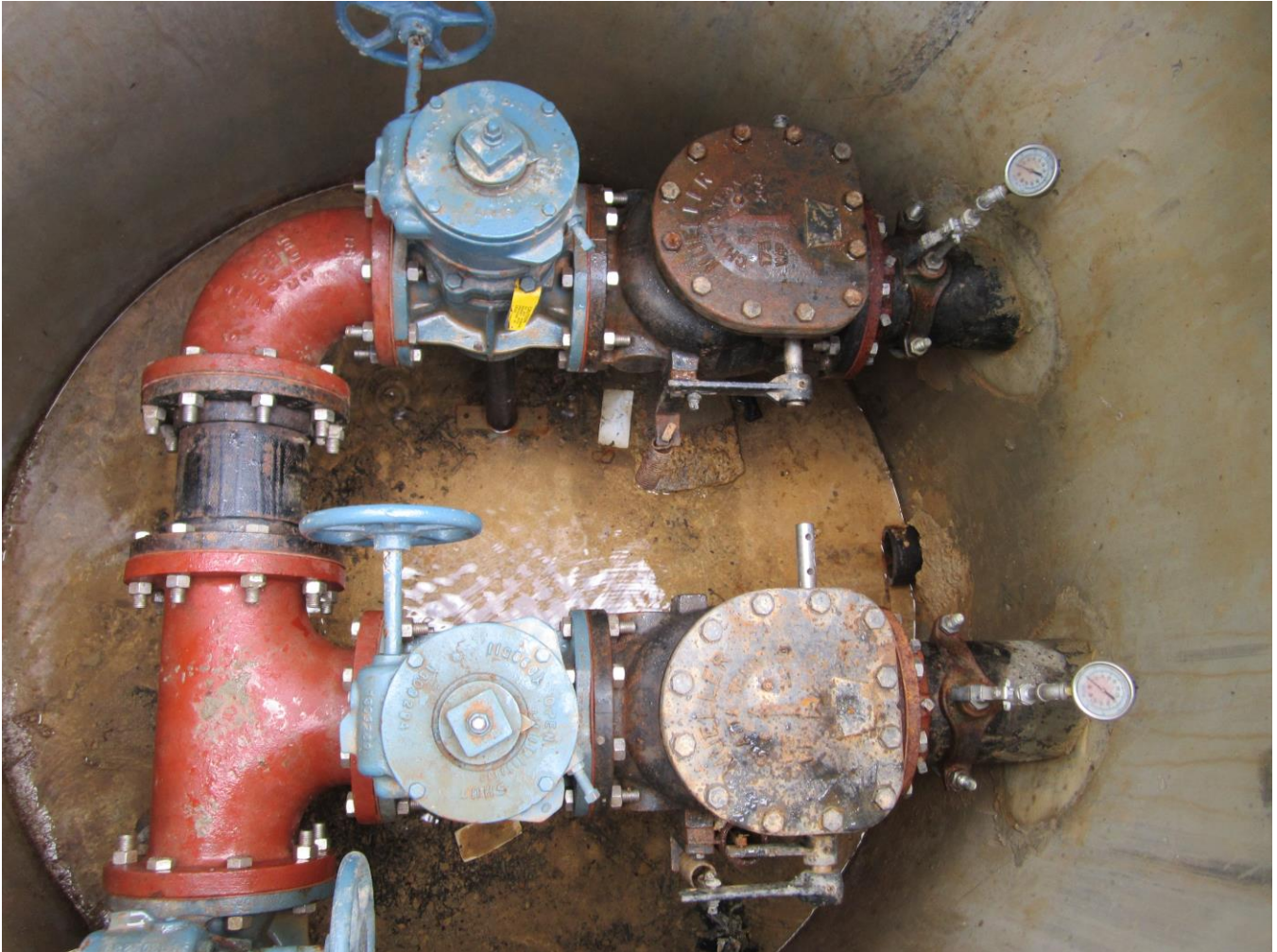
PHOTO 2: VALVE PIT PIPING AND PRESSURE GAUGES
