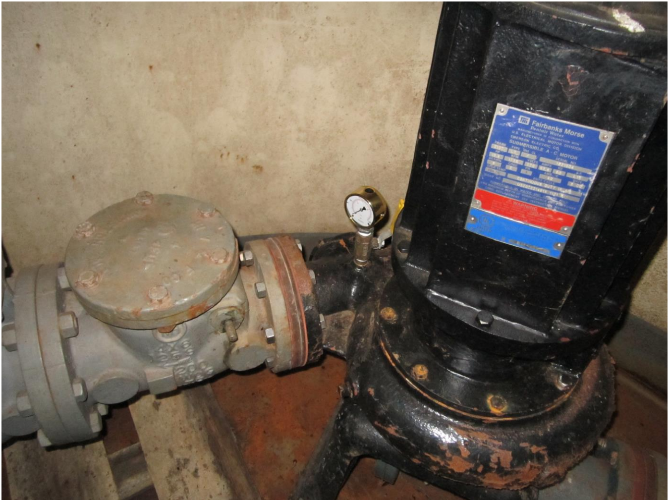
PHOTO 2: PUMP AND PRESSURE GAUGE
