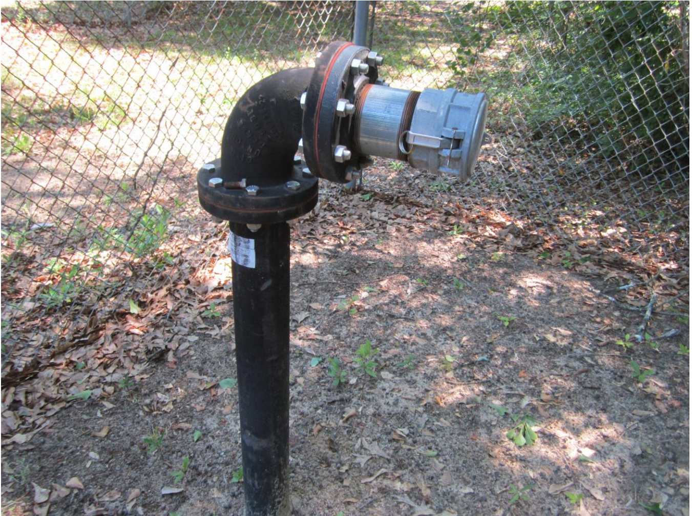
PHOTO 2: BYPASS PUMPING CONNECTION
