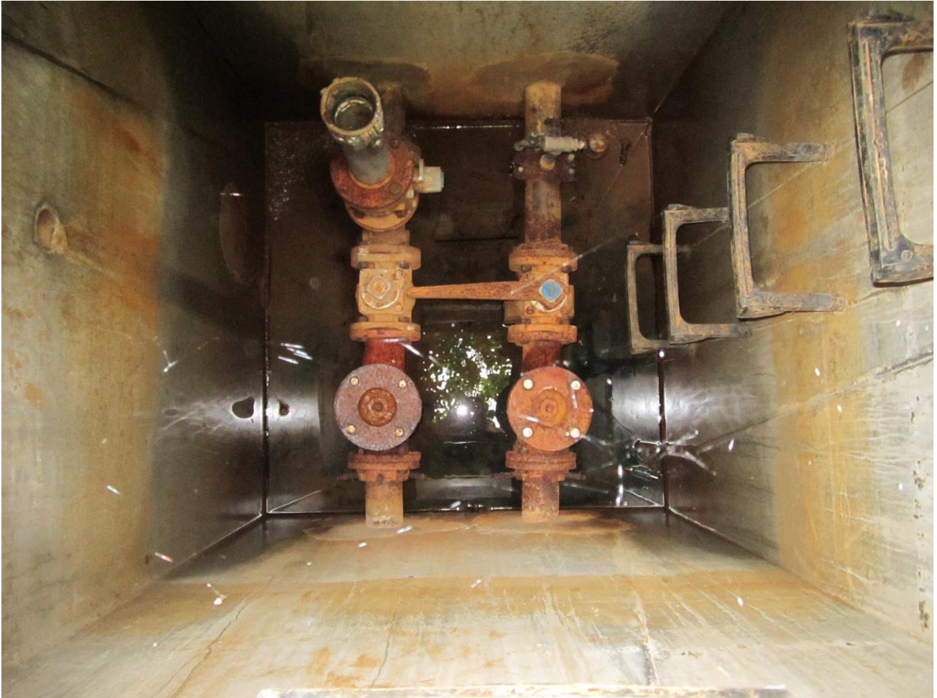
PHOTO 2: VALVE VAULT PIPING, BYPASS AND PRESSURE GAUGE
