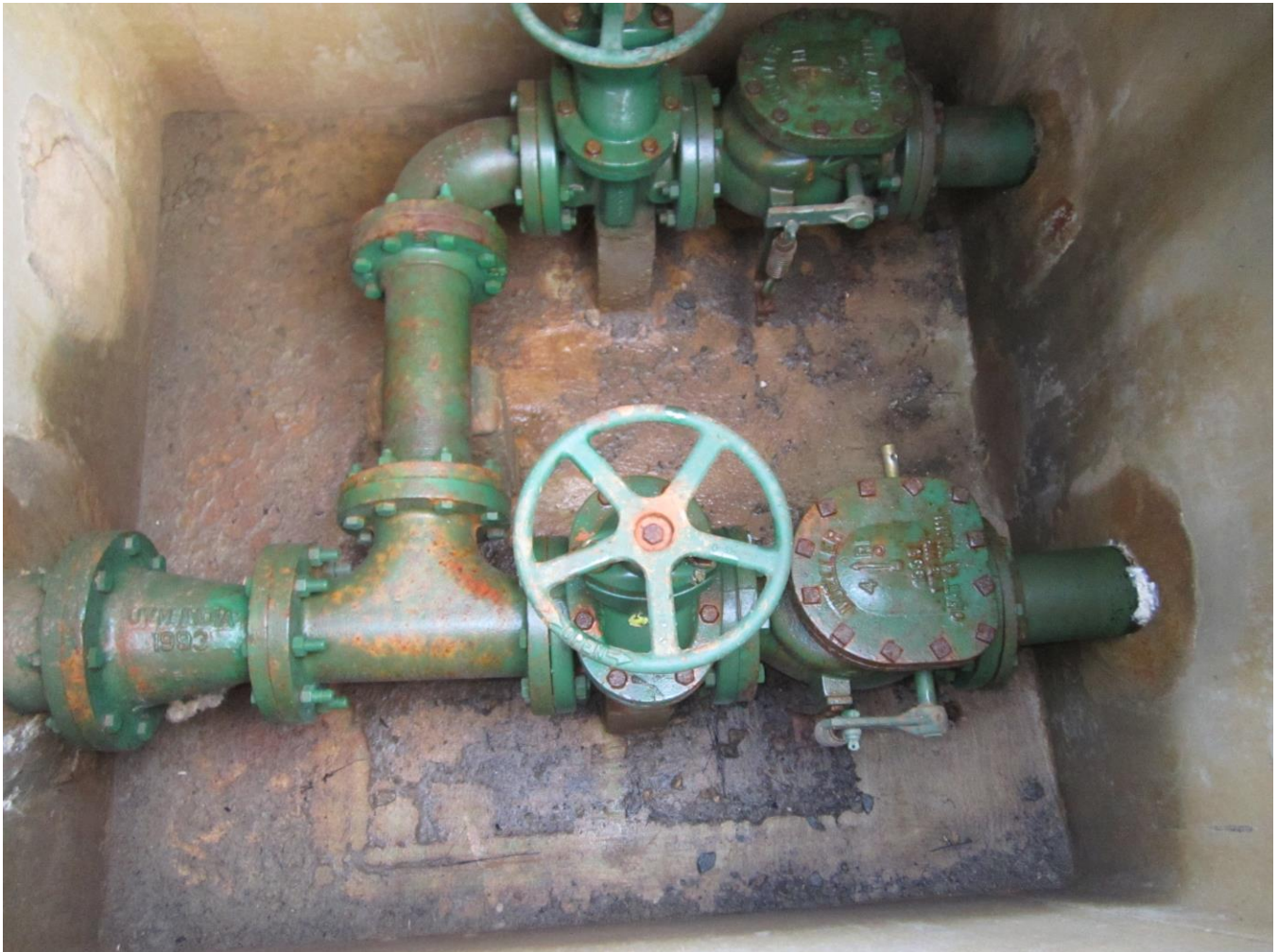
PHOTO 2: VALVE PIT PIPING
