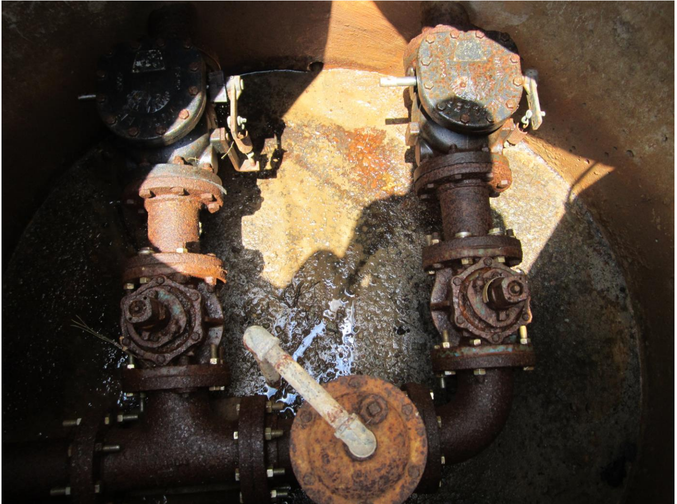
PHOTO 2: VALVE VAULT PIPING
