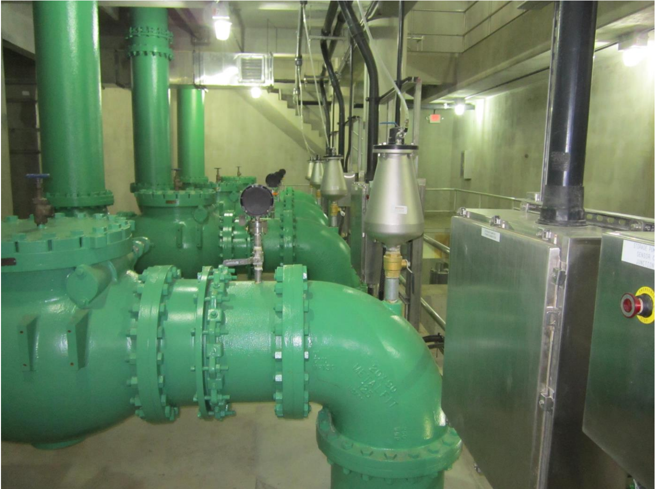
PHOTO 2: DISCHARGE HEADER WITH GAUGES AND ARV'S
