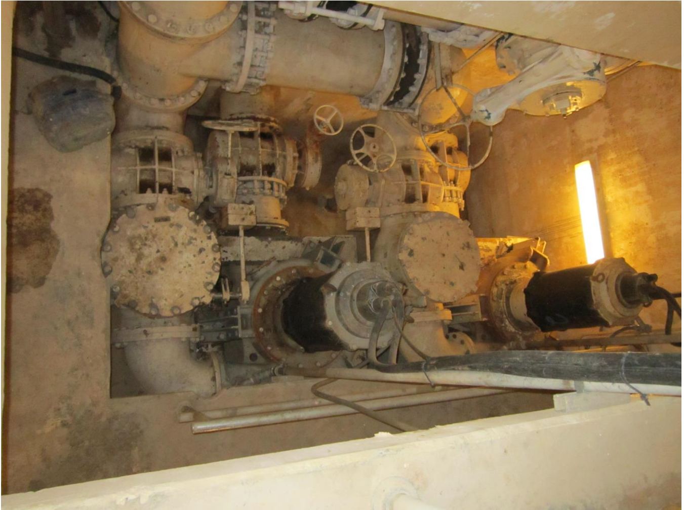
PHOTO 2: 150 Hp PUMPS AND PIPING
