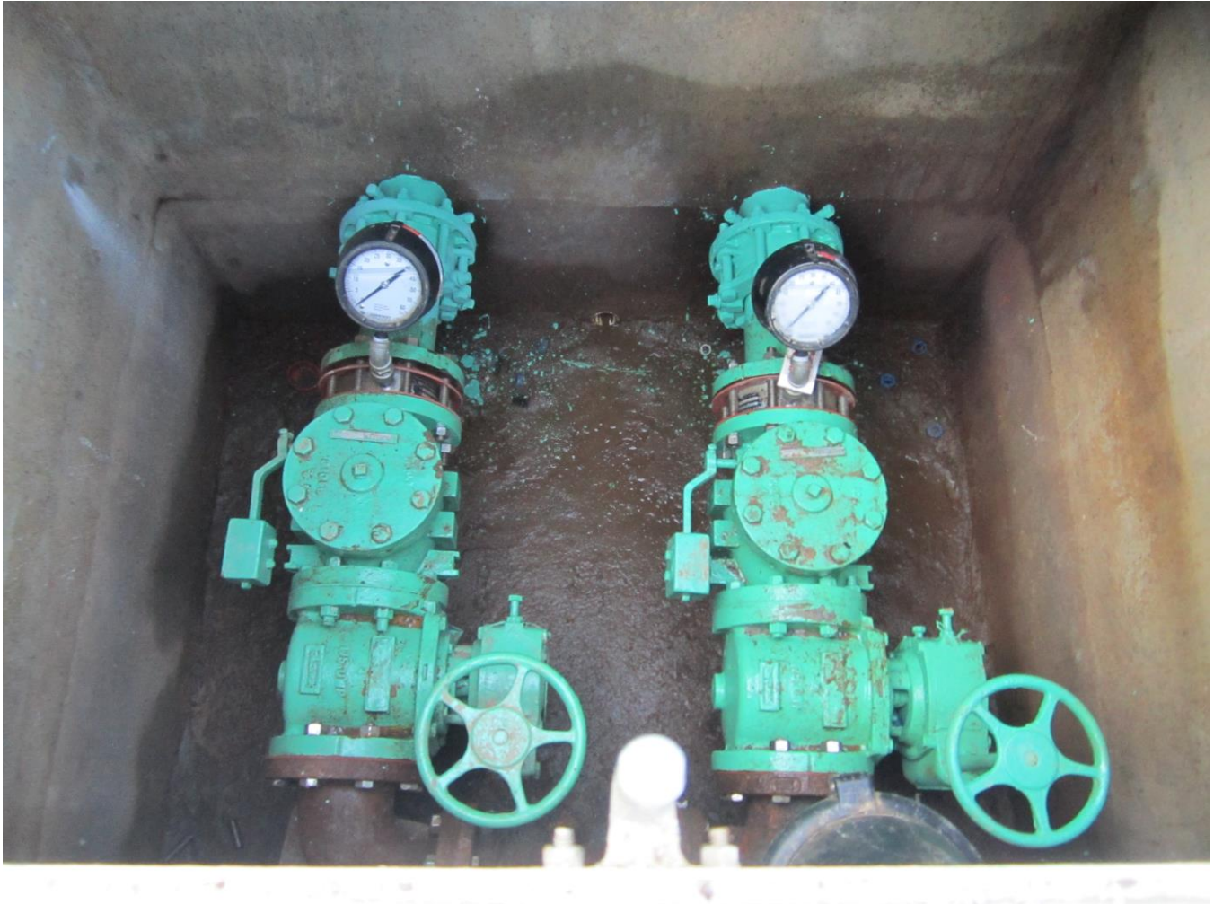
PHOTO 2: VALVE PIT PIPING AND PRESSURE GAUGES
