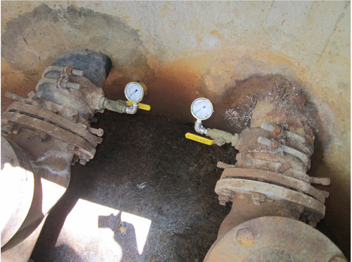
PHOTO 2: VALVE PIT PIPING AND PRESSURE GAUGES
