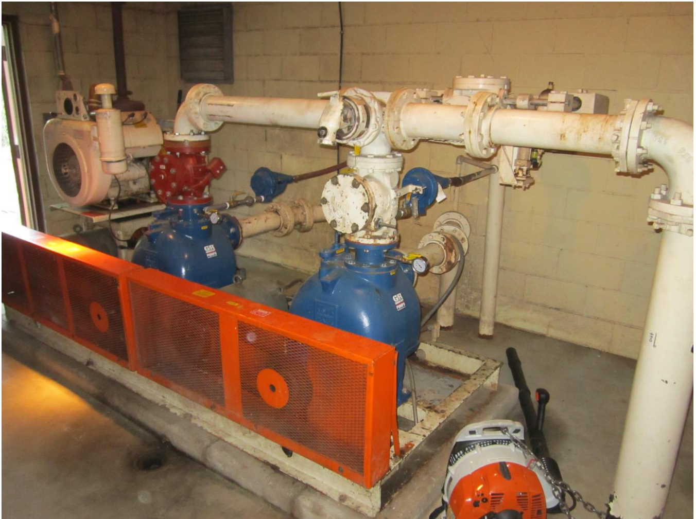
PHOTO 2: PUMPS AND PIPING
