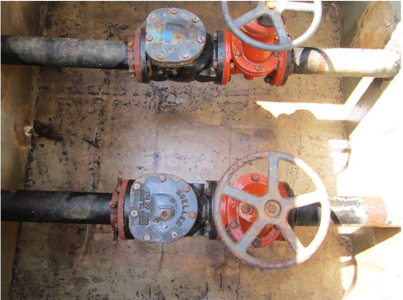
PHOTO 2: VALVE VAULT PIPING
