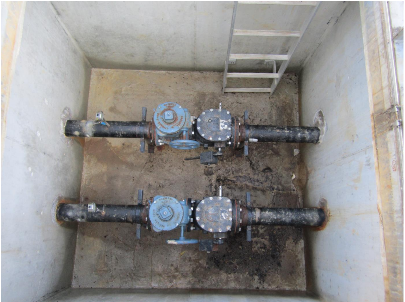
PHOTO 2: VALVE PIT PIPING AND PRESSURE GAUGES
