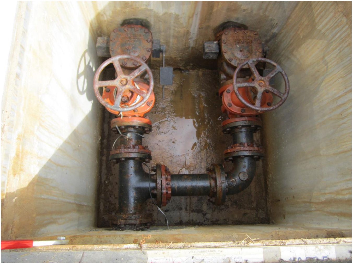
PHOTO 2: VALVE PIT PIPING
