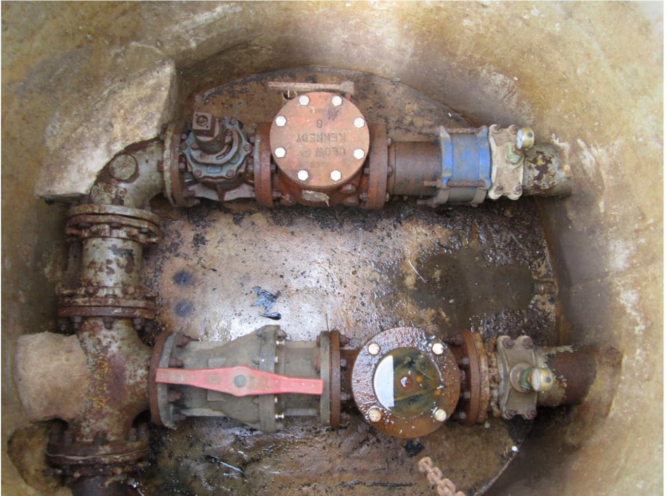
PHOTO 2: VALVE PIT PIPING AND PRESSURE GAUGES
