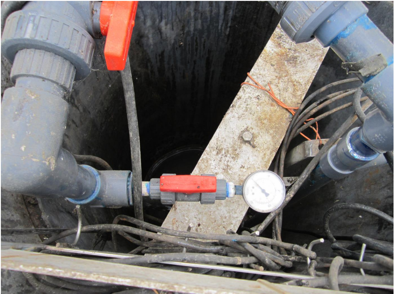
PHOTO 2: WETWELL INTERIOR AND PRESSURE GAUGE
