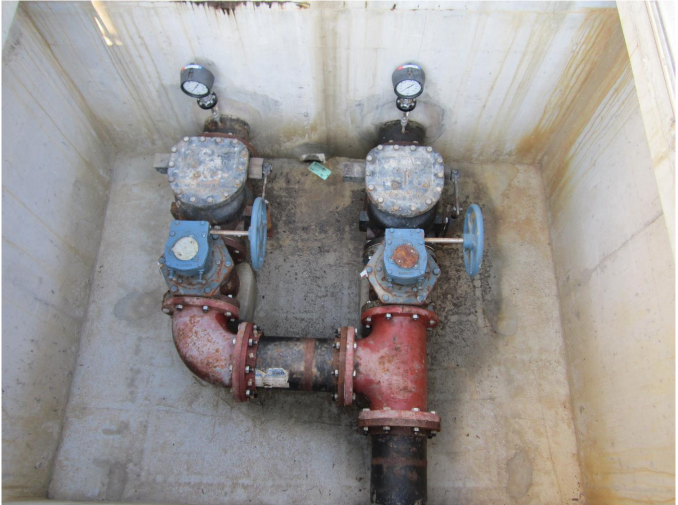
PHOTO 2: VALVE PIT PIPING AND PRESSURE GAUGES
