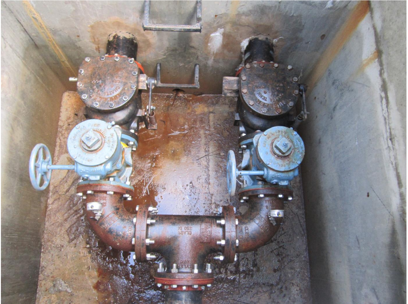
PHOTO 2: VALVE PIT PIPING
