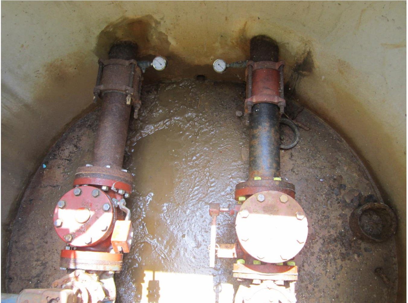
PHOTO 2: VALVE PIT PIPING AND PRESSURE GAUGES
