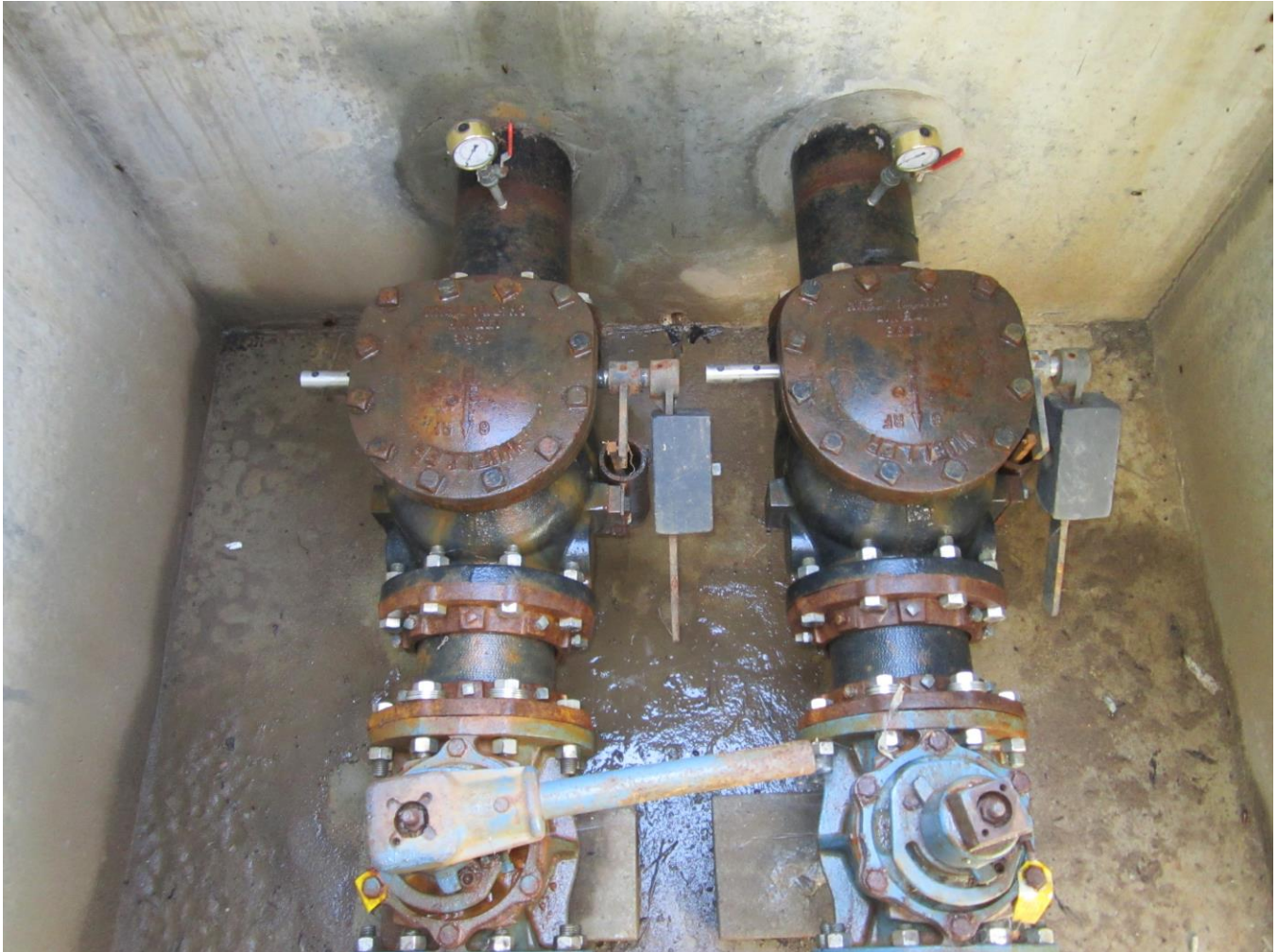
PHOTO 2: VALVE PIT PIPING AND PRESSURE GAUGES
