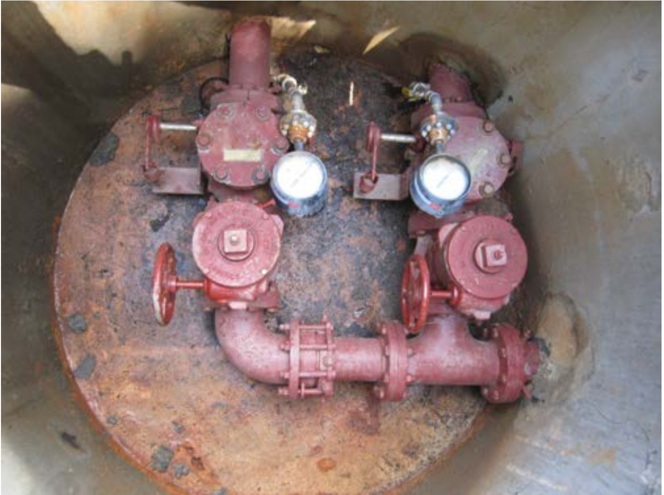
PHOTO 2: VALVE PIT PIPING AND PRESSURE GAUGES
