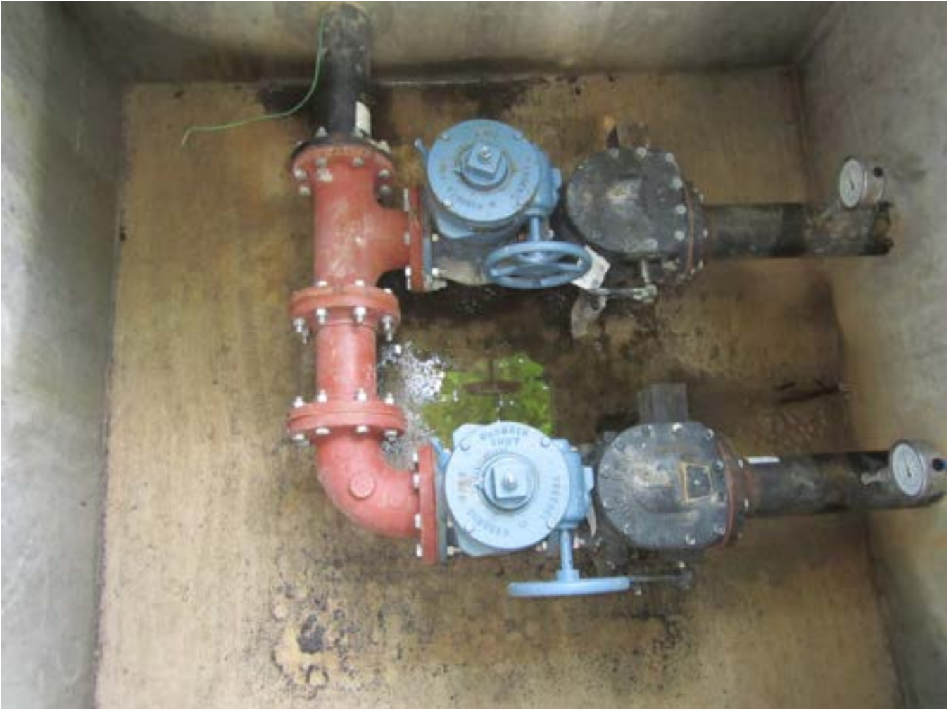
PHOTO 2: VALVE PIT PIPING AND PRESSURE GAUGES
