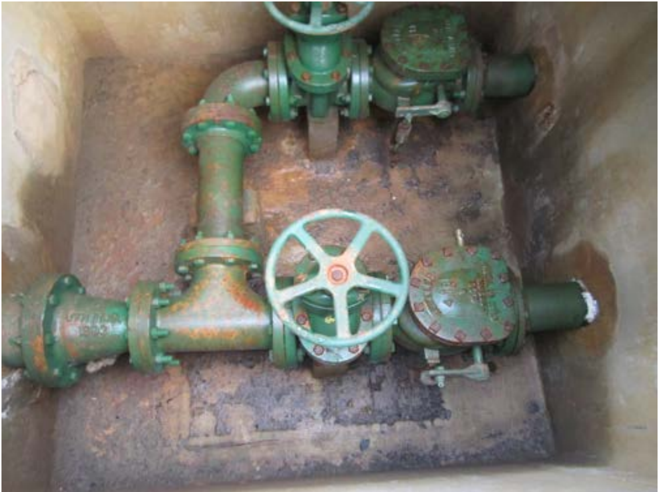
PHOTO 2: VALVE PIT PIPING
