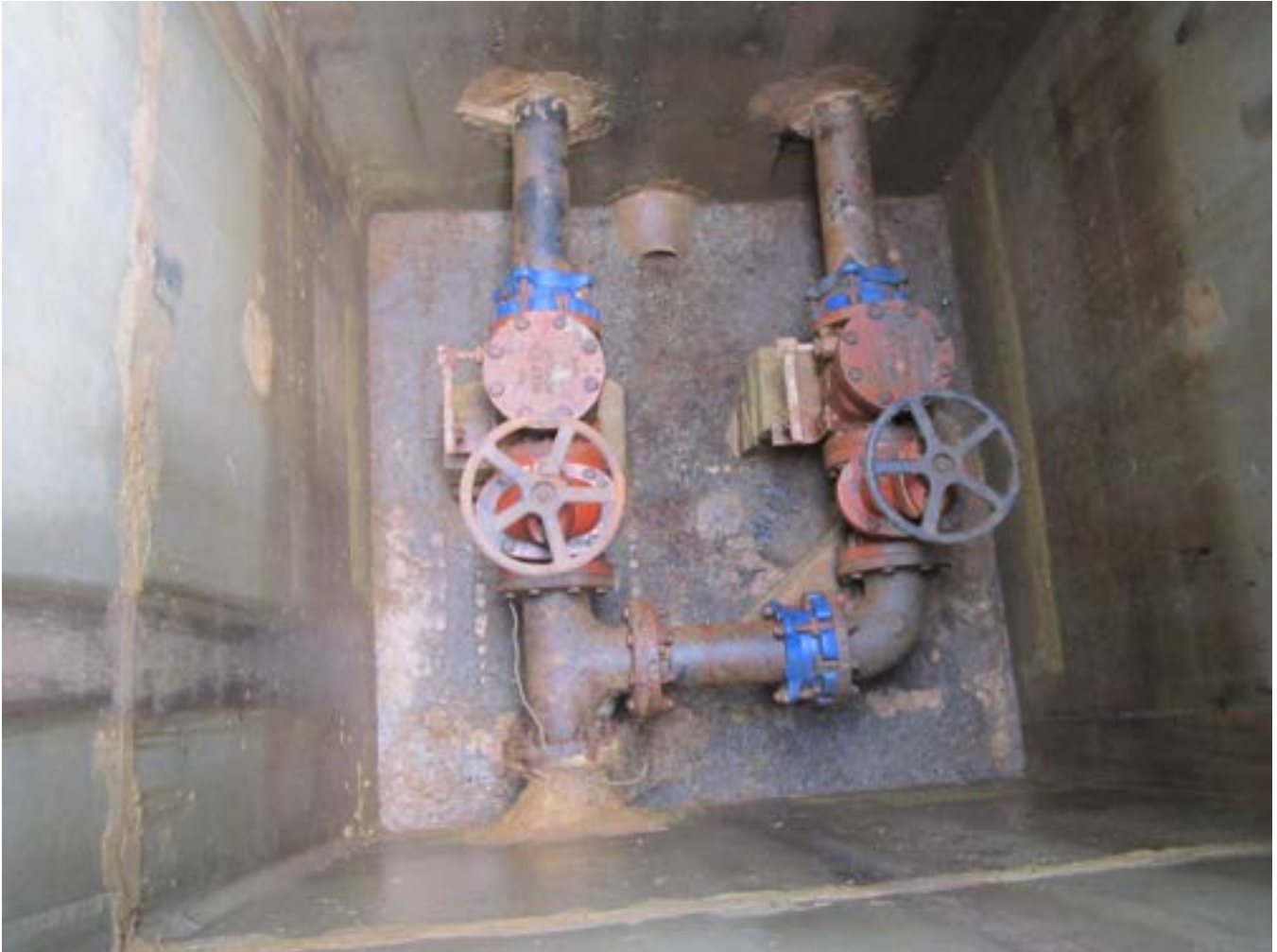
PHOTO 2: VALVE VAULT PIPING
