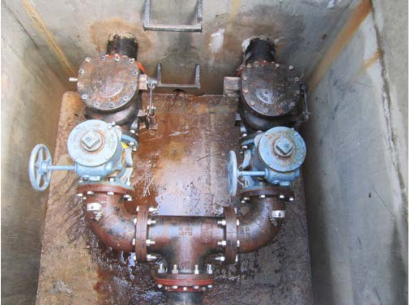
PHOTO 2: VALVE PIT PIPING
