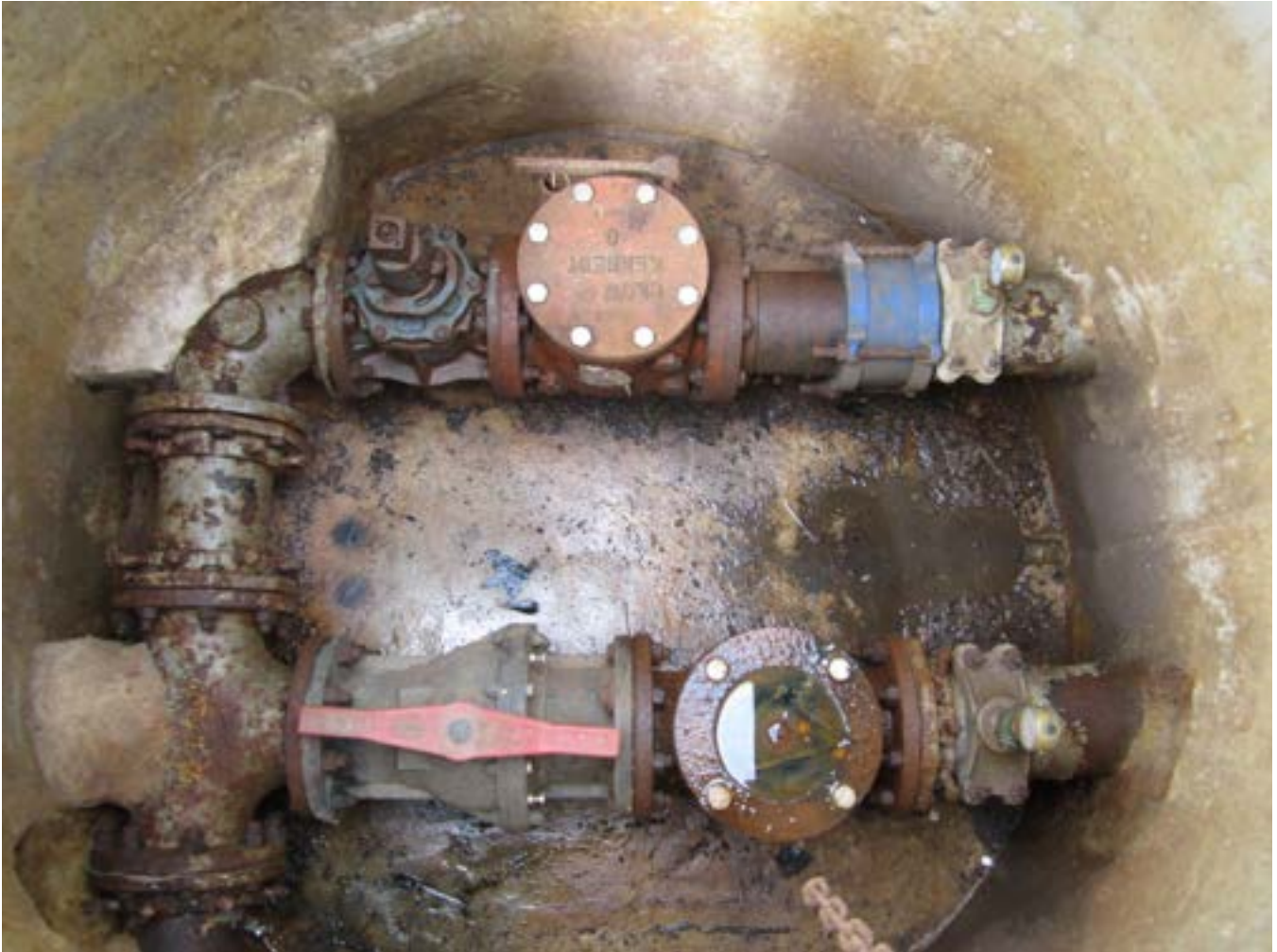
PHOTO 2: VALVE PIT PIPING AND PRESSURE GAUGES
