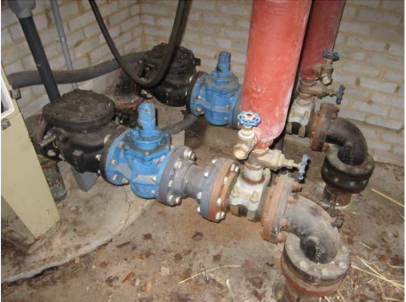
PHOTO 2: DISCHARGE PIPING HEADER
