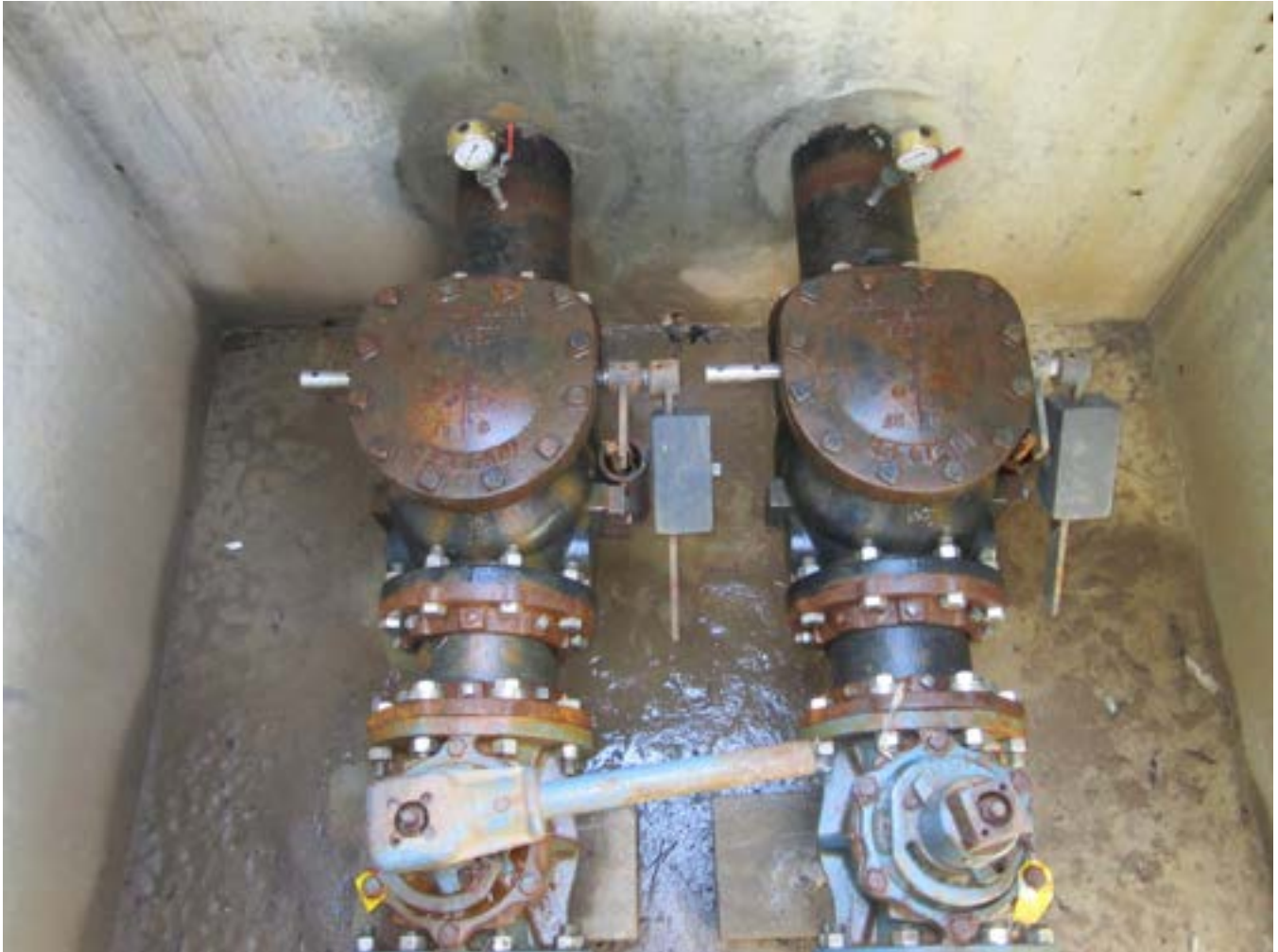
PHOTO 2: VALVE PIT PIPING AND PRESSURE GAUGES
