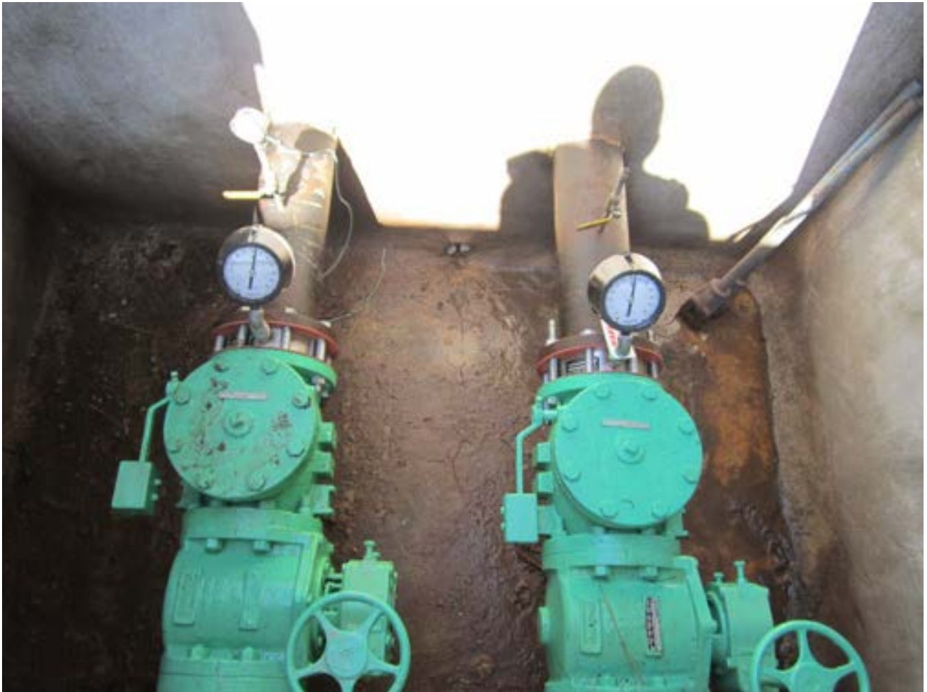
PHOTO 2: VALVE PIT PIPING AND PRESSURE GAUGES
