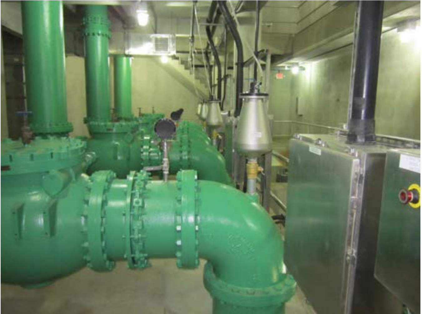
PHOTO 2: DISCHARGE HEADER WITH GAUGES AND ARV'S
