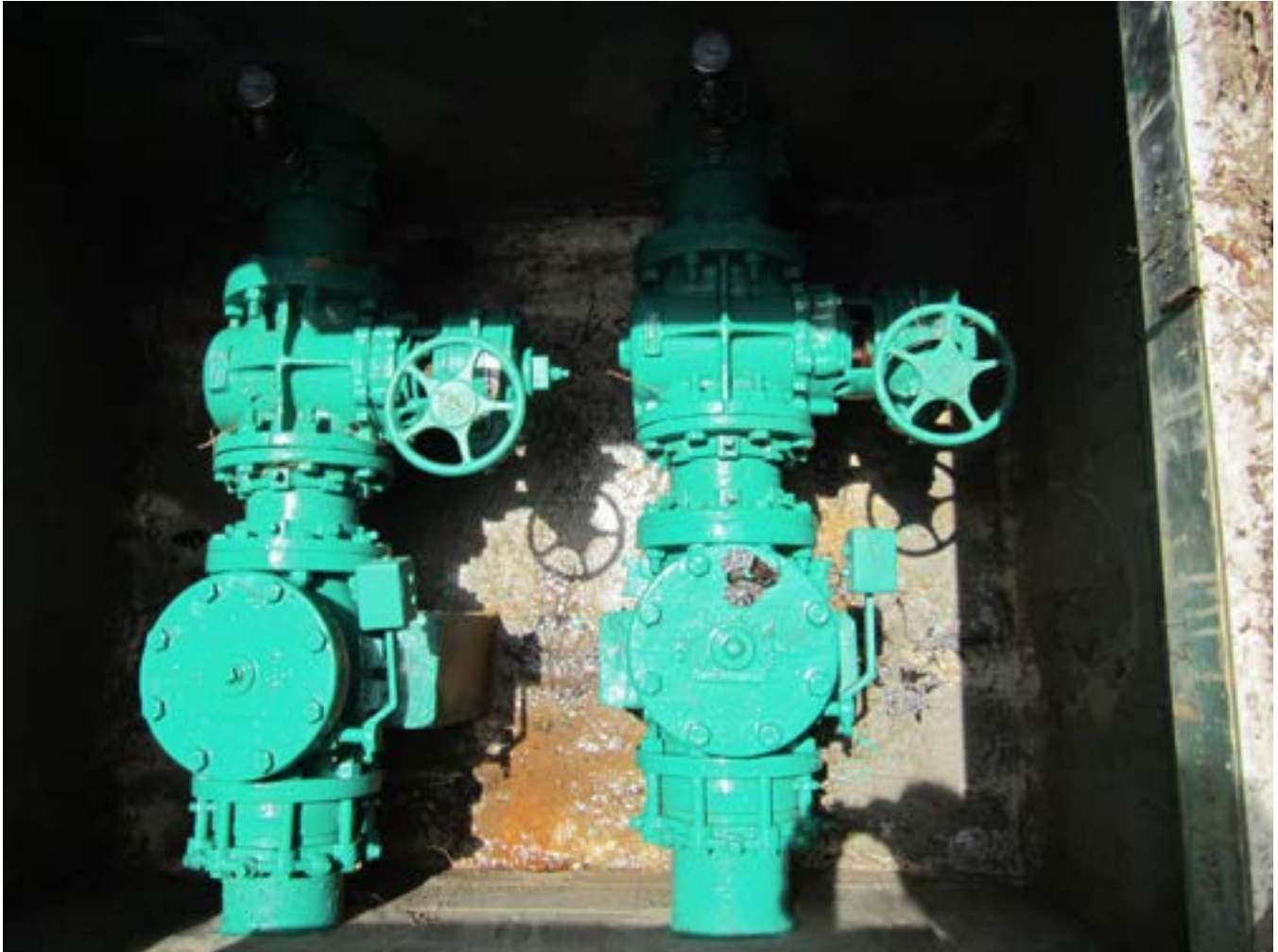
PHOTO 2: VALVE PIT PIPING AND PRESSURE GAUGES
