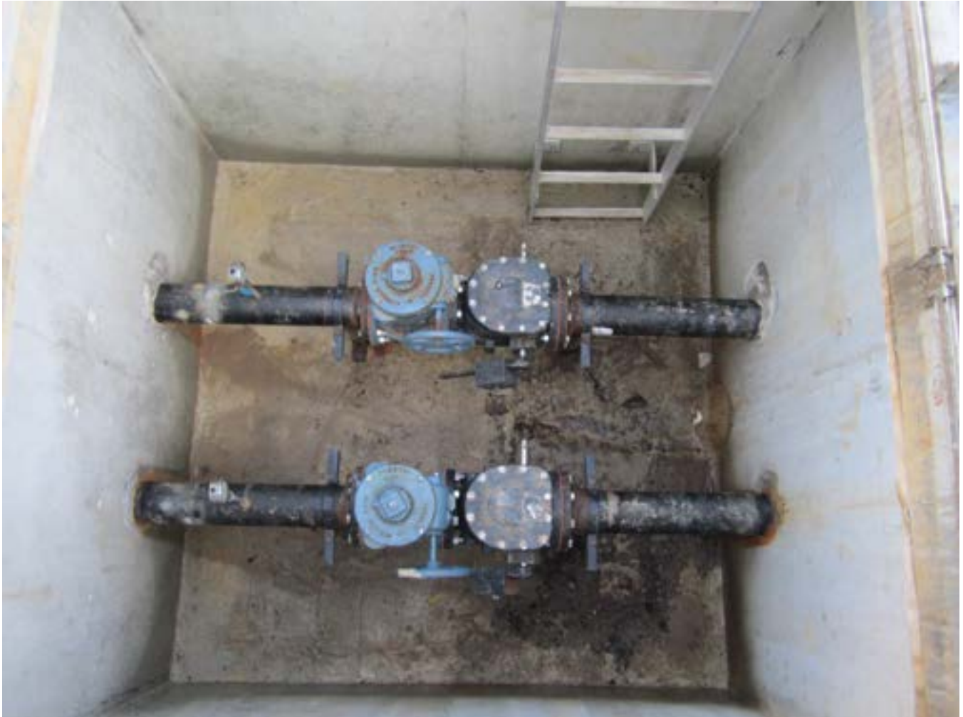
PHOTO 2: VALVE PIT PIPING AND PRESSURE GAUGES
