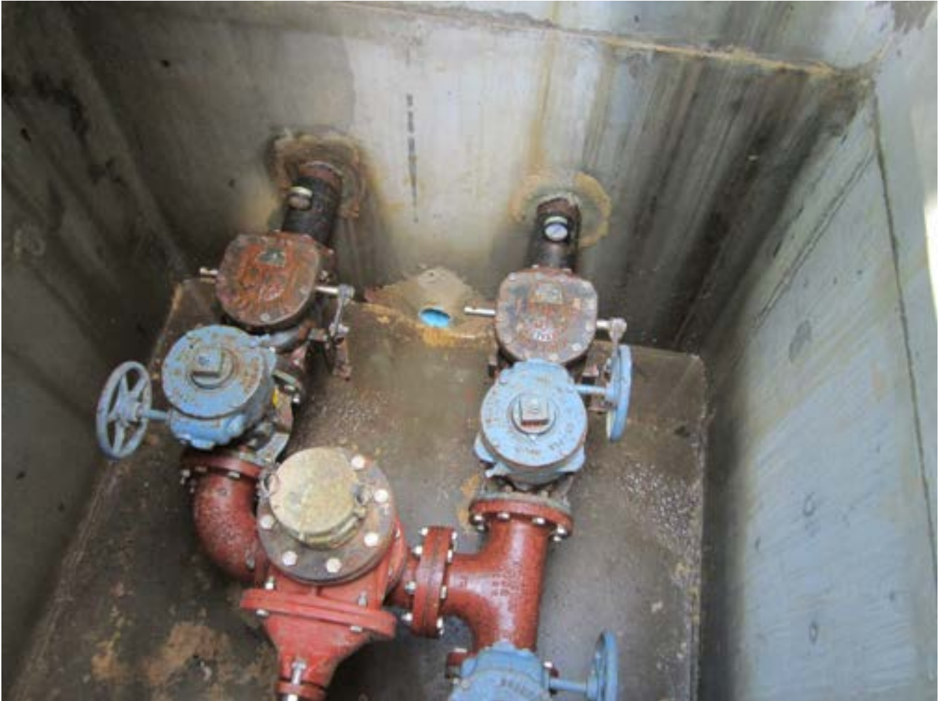
PHOTO 2: VALVE VAULT PIPING, BYPASS AND PRESSURE GAUGE
