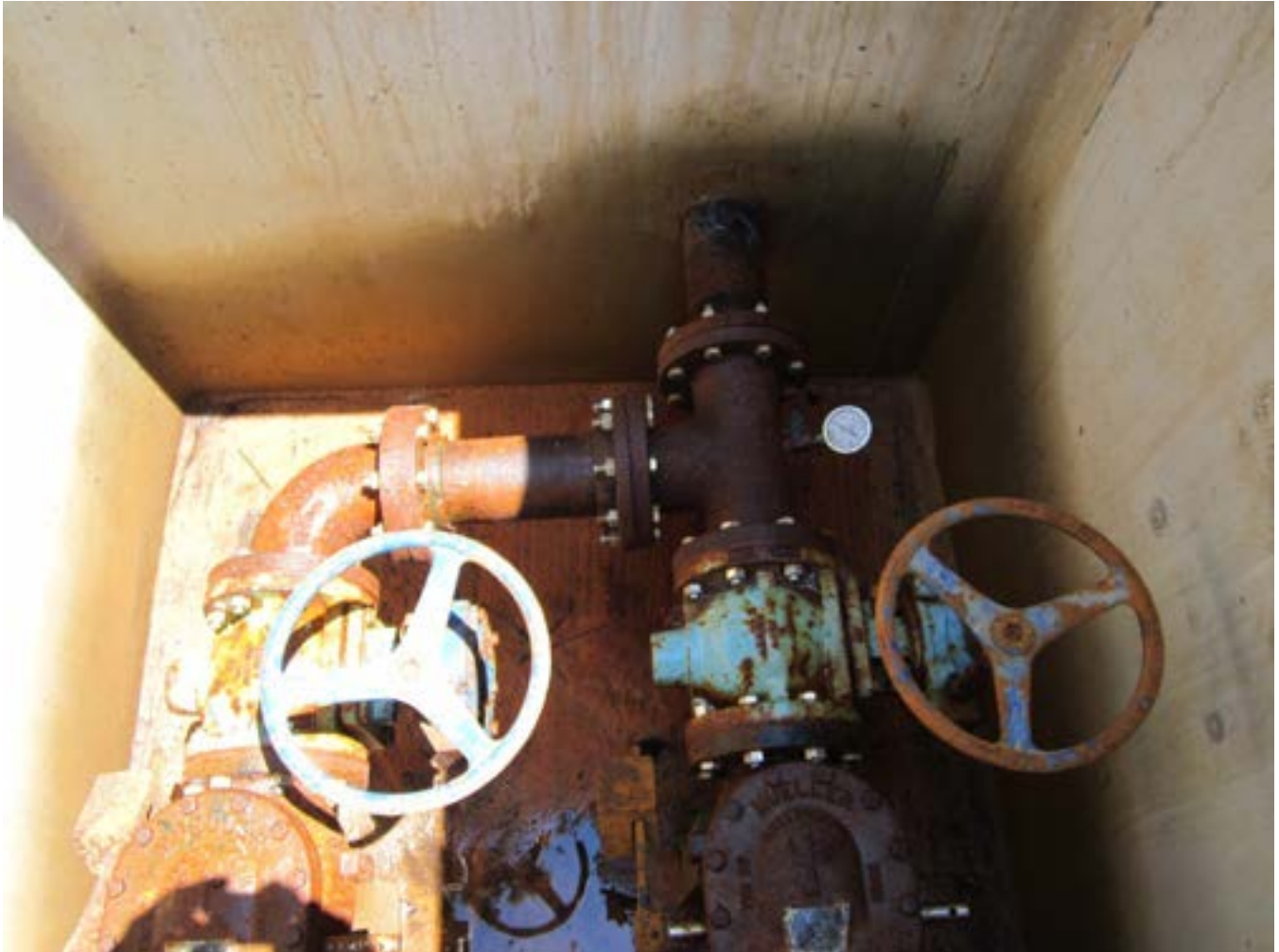
PHOTO 2: DISCHARGE HEADER PRESSURE GAUGE
