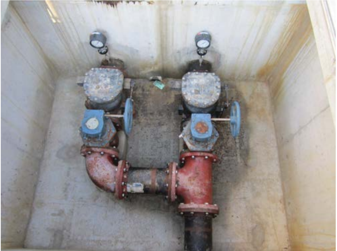
PHOTO 2: VALVE PIT PIPING AND PRESSURE GAUGES
