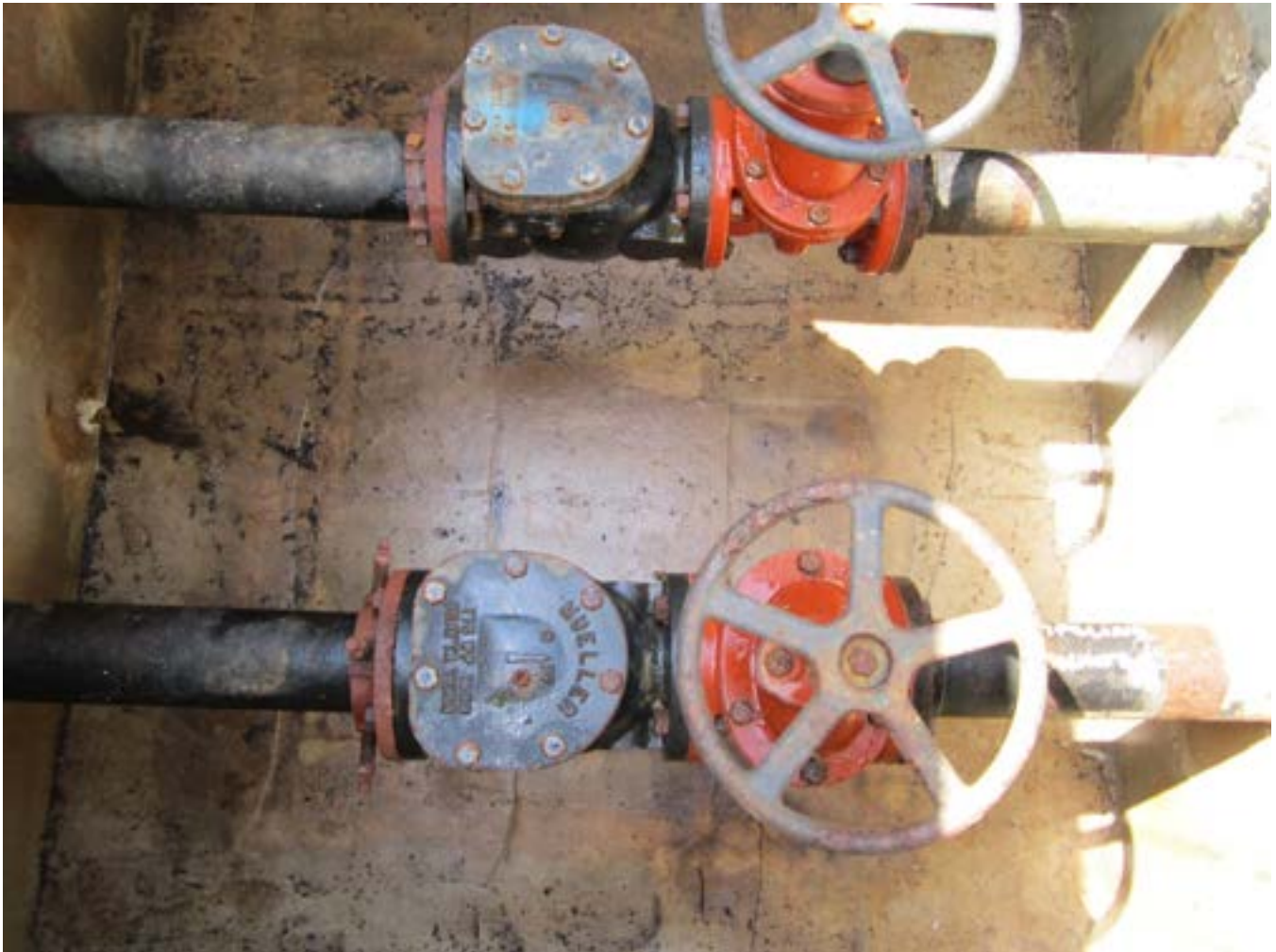
PHOTO 2: VALVE VAULT PIPING
