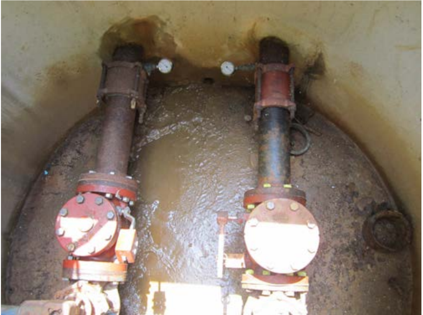
PHOTO 2: VALVE PIT PIPING AND PRESSURE GAUGES
