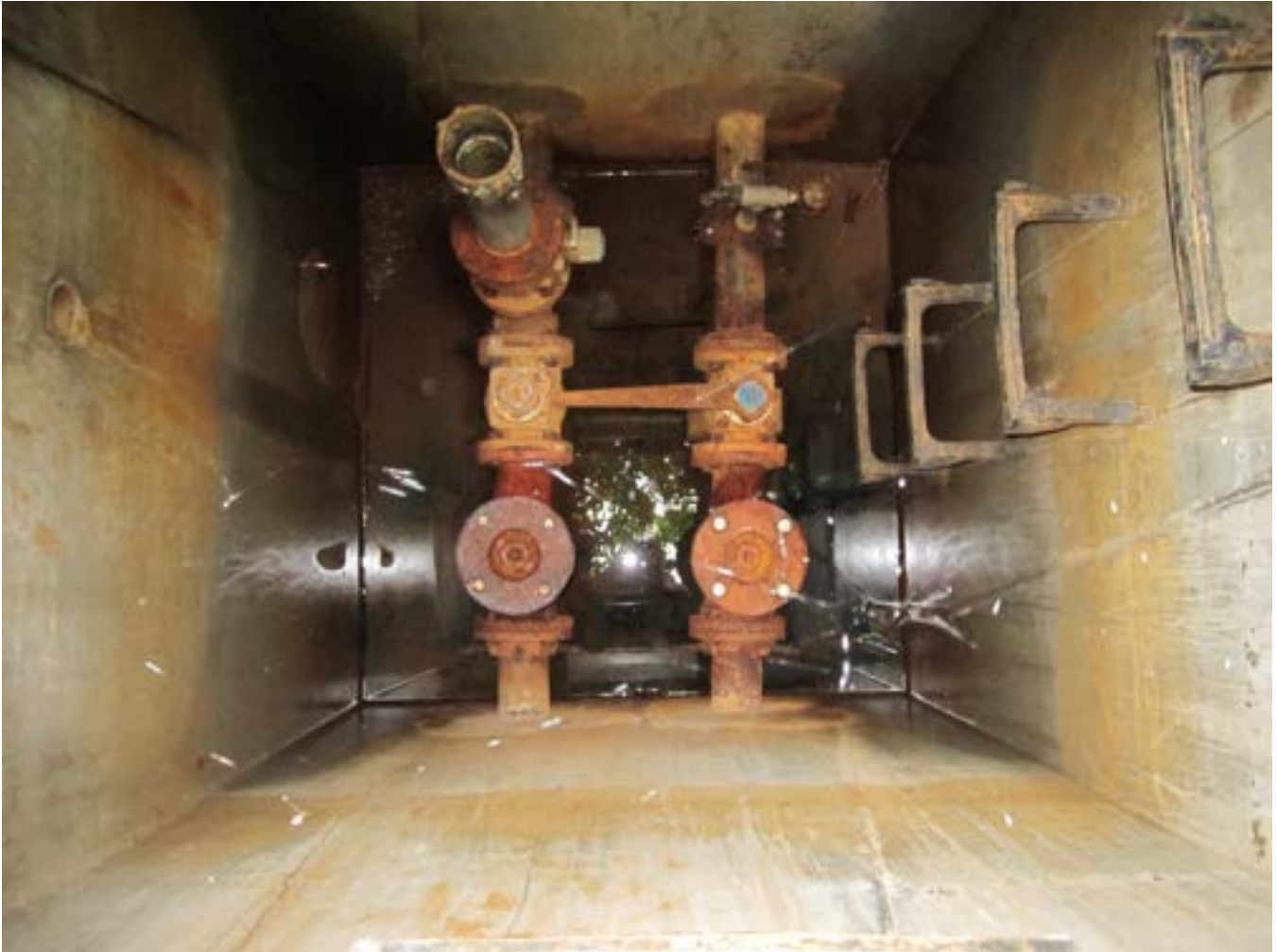
PHOTO 2: VALVE VAULT PIPING, BYPASS AND PRESSURE GAUGE
