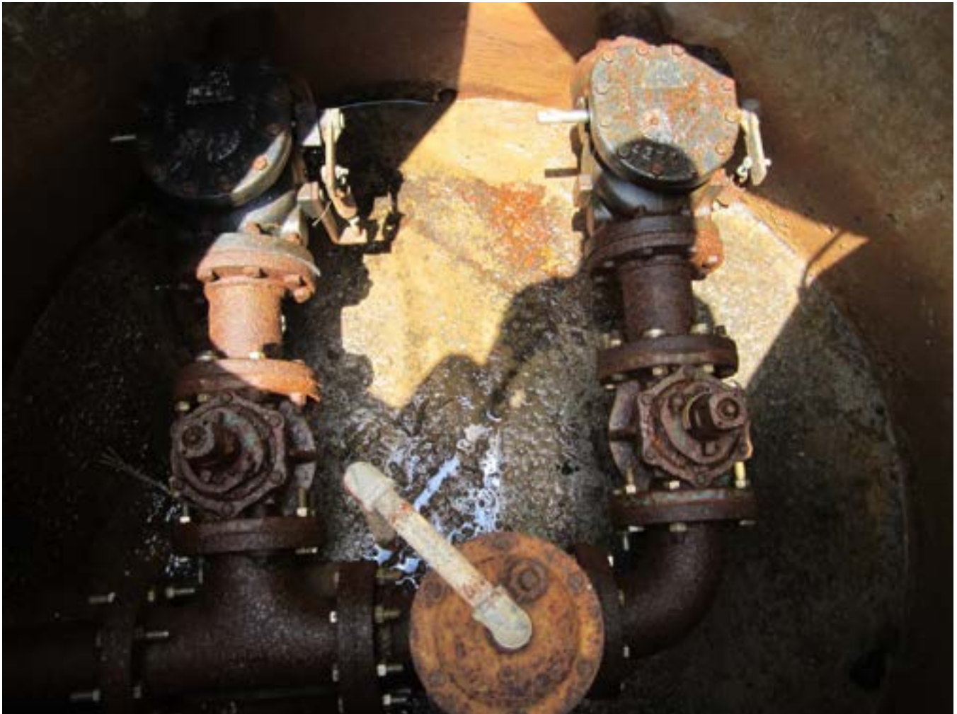
PHOTO 2: VALVE VAULT PIPING
