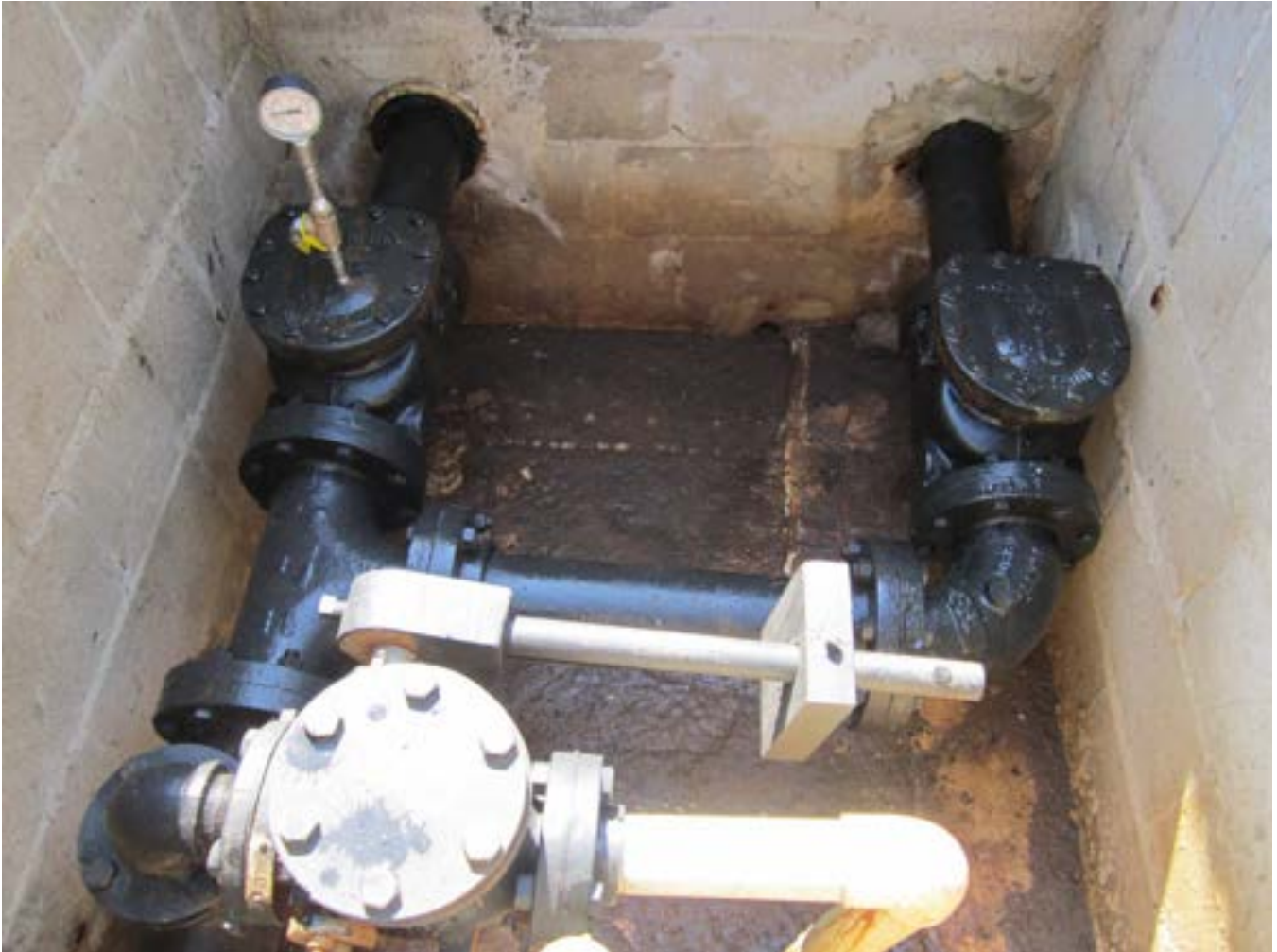
PHOTO 2: VALVE PIT PIPING AND PRESSURE GAUGE
