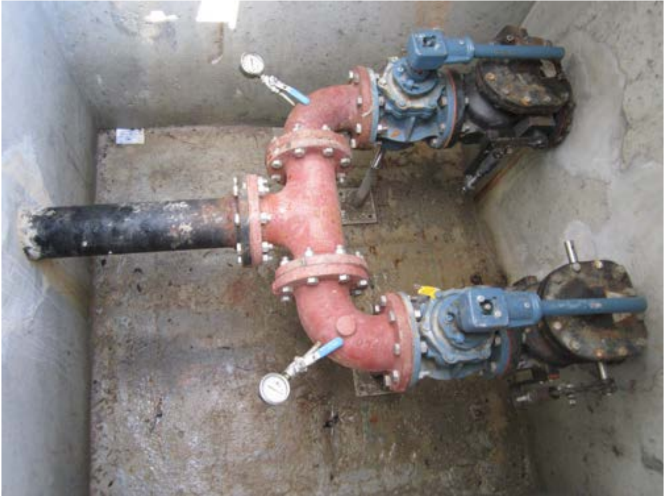
PHOTO 2: VALVE PIT PIPING AND PRESSURE GAUGES
