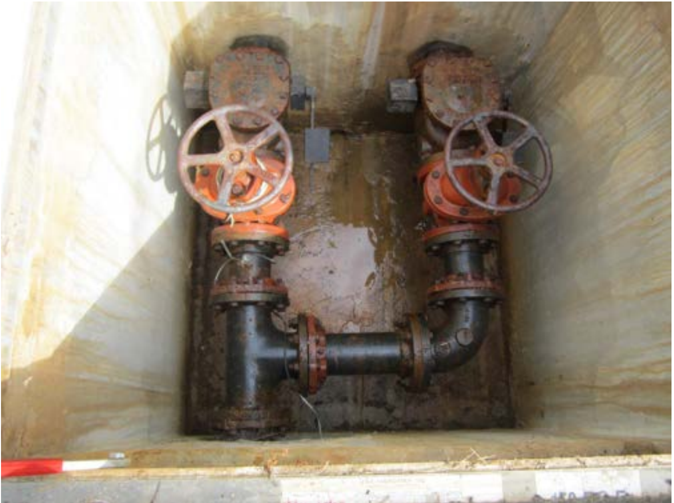
PHOTO 2: VALVE PIT PIPING
