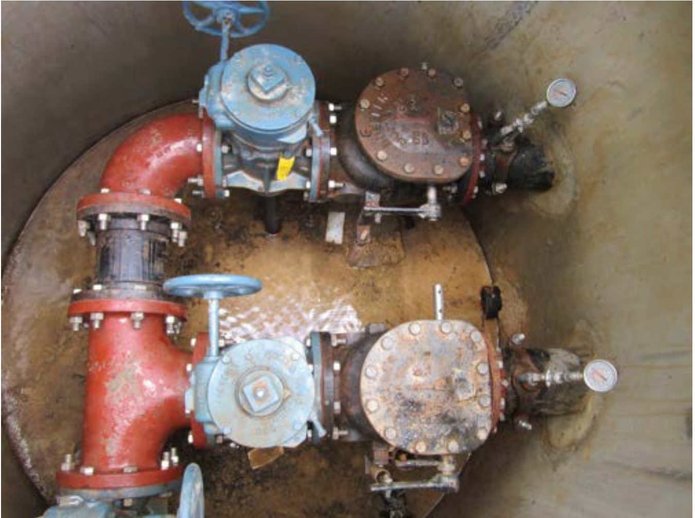
PHOTO 2: VALVE PIT PIPING AND PRESSURE GAUGES
