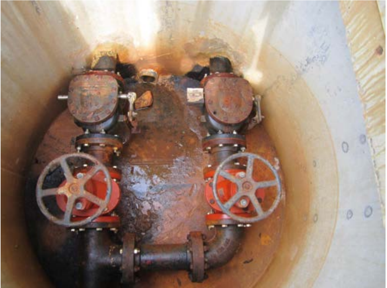
PHOTO 2: VALVE VAULT PIPING
