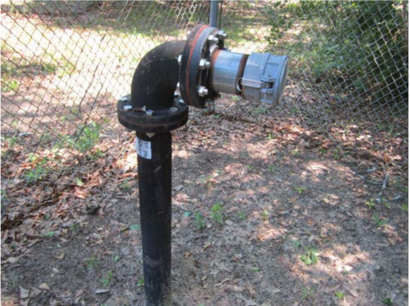
PHOTO 2: BYPASS PUMPING CONNECTION
