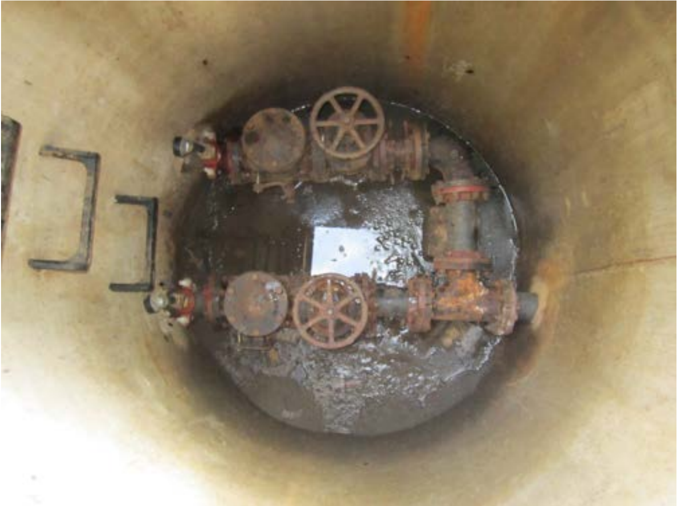
PHOTO 2: VALVE PIT PIPING AND PRESSURE GAUGES
