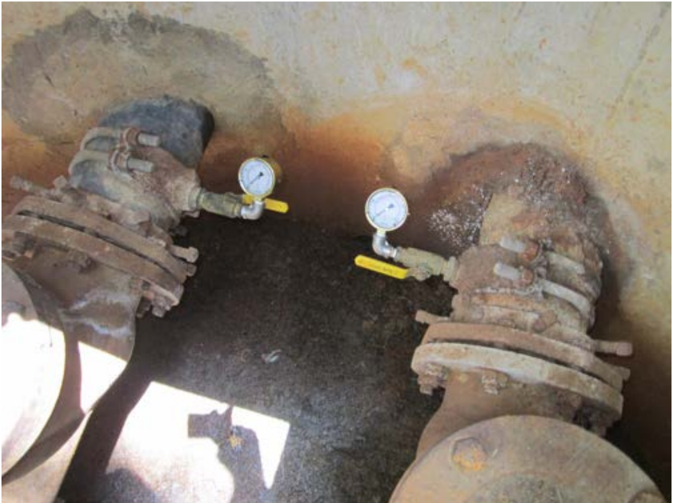
PHOTO 2: VALVE PIT PIPING AND PRESSURE GAUGES
