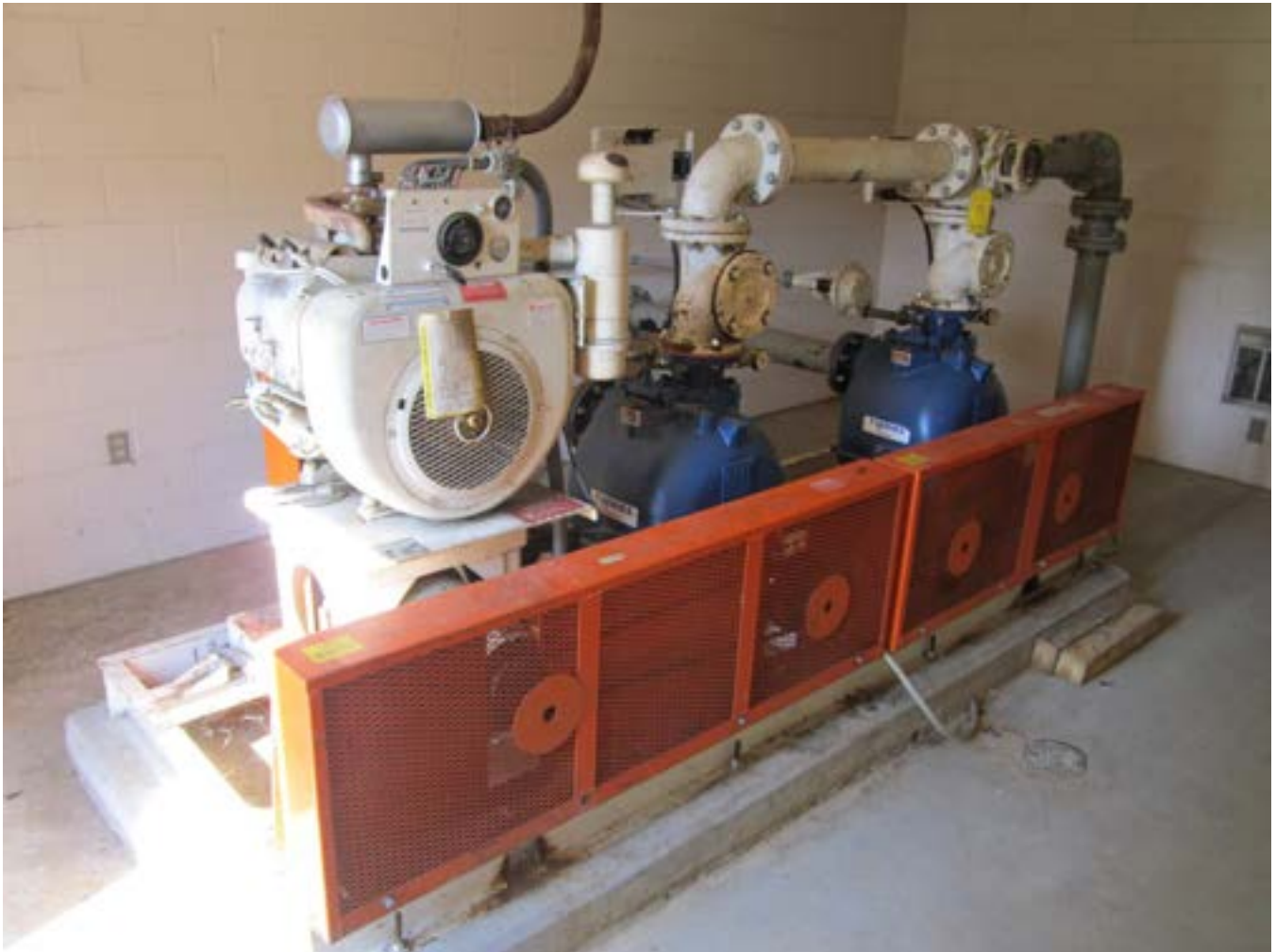
PHOTO 2: SELF PRIMING PUMPS, PIPING AND BACK UP MOTOR
