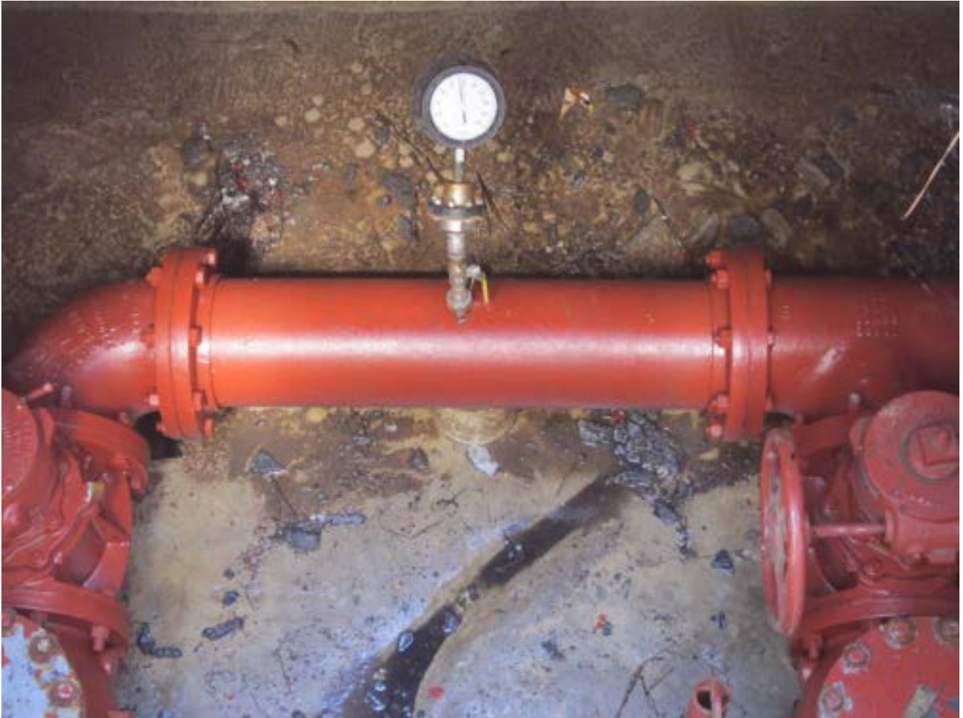
PHOTO 2: DISCHARGE HEADER PRESSURE GAUGE
