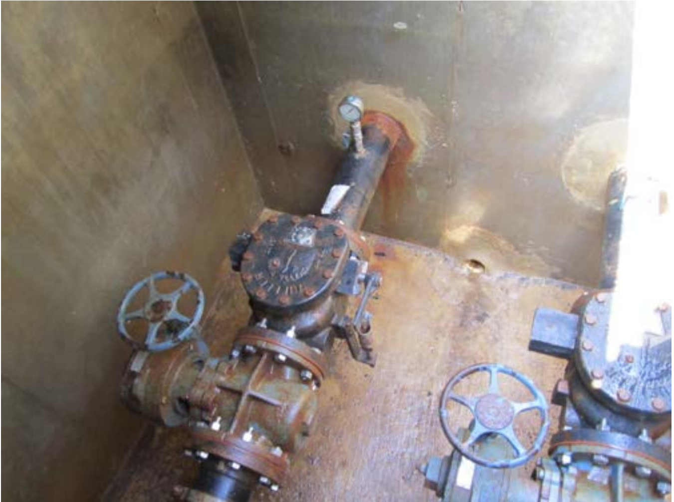
PHOTO 2: VALVE PIT PIPING AND PRESSURE GAUGE
