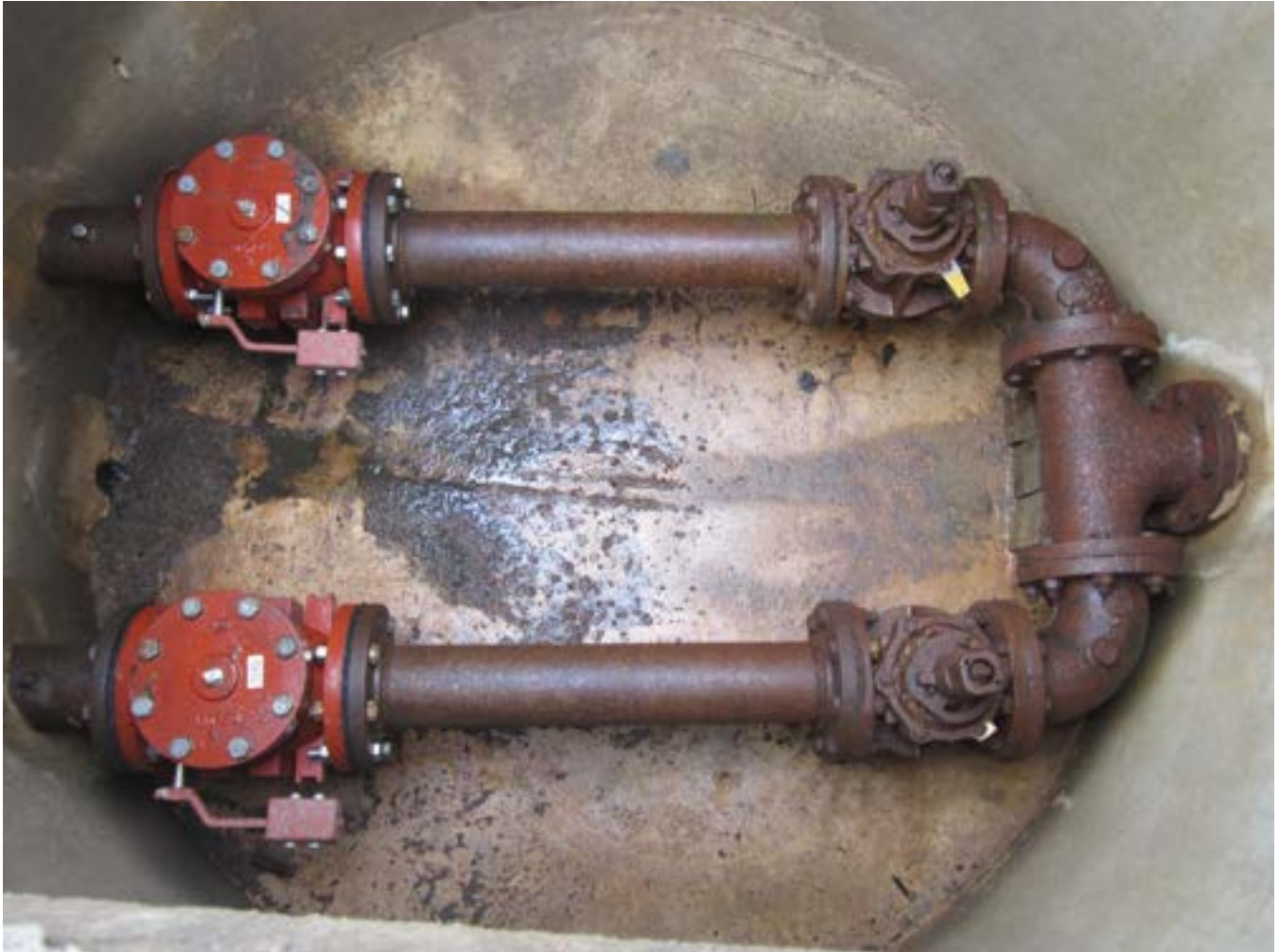
PHOTO 2: VALVE PIT PIPING
