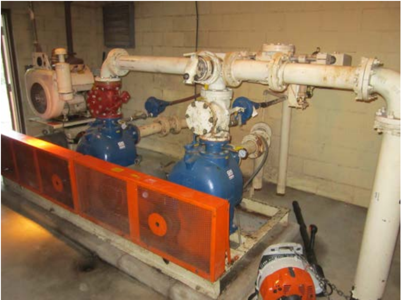
PHOTO 2: PUMPS AND PIPING
