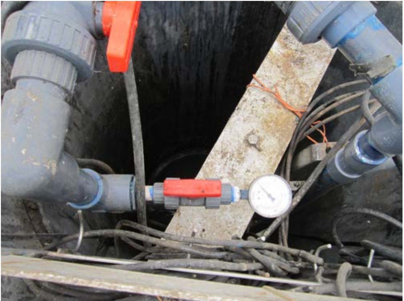
PHOTO 2: WETWELL INTERIOR AND PRESSURE GAUGE
