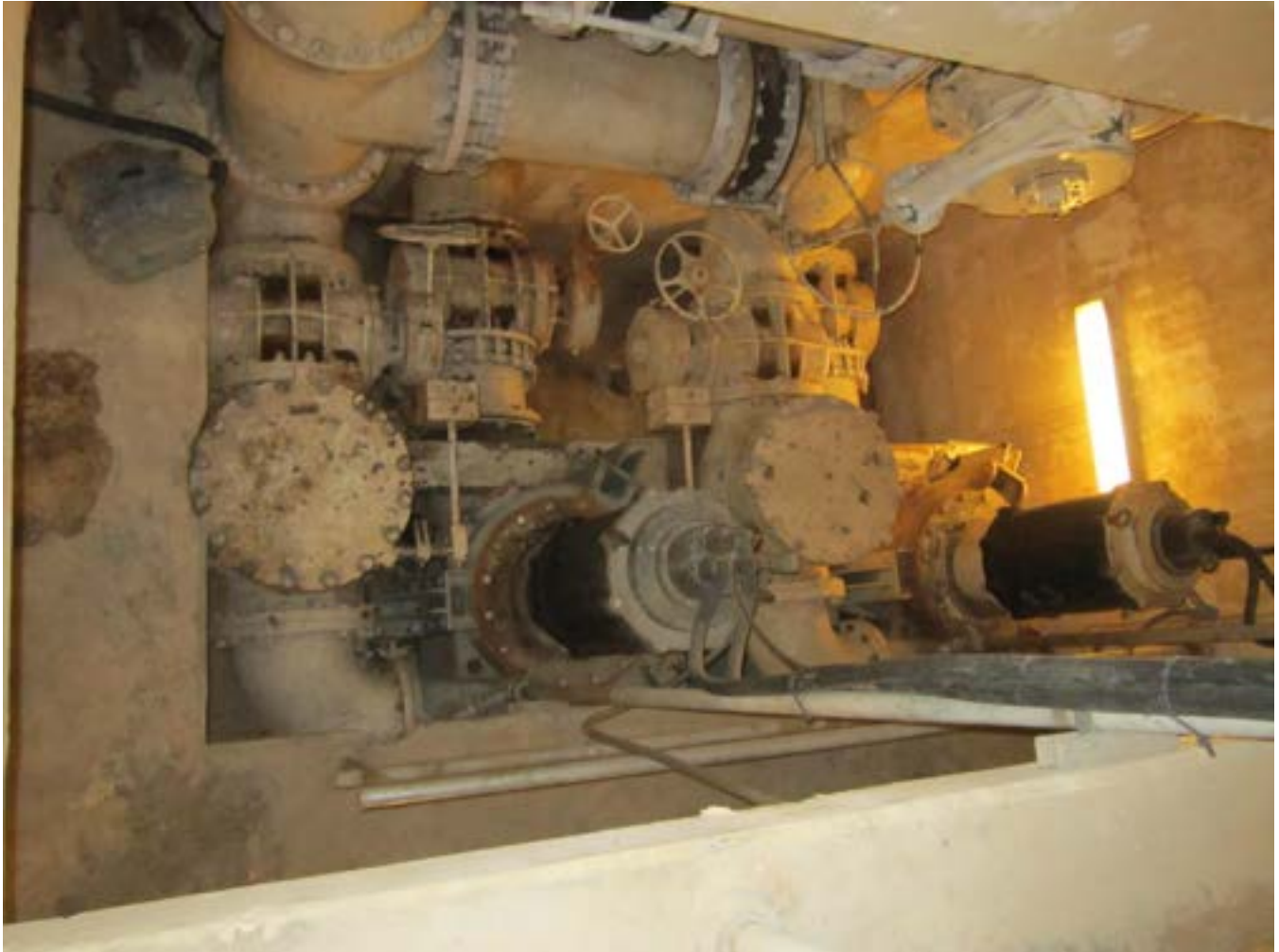
PHOTO 2: 150 Hp PUMPS AND PIPING
