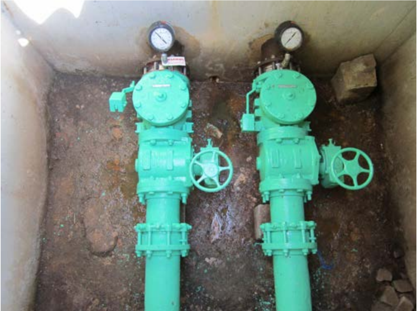
PHOTO 2: VALVE PIT PIPING AND PRESSURE GAUGES
