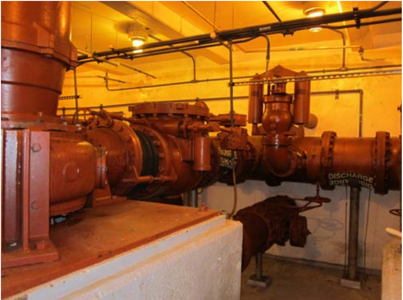
PHOTO 2: DISCHARGE HEADER PIPING
