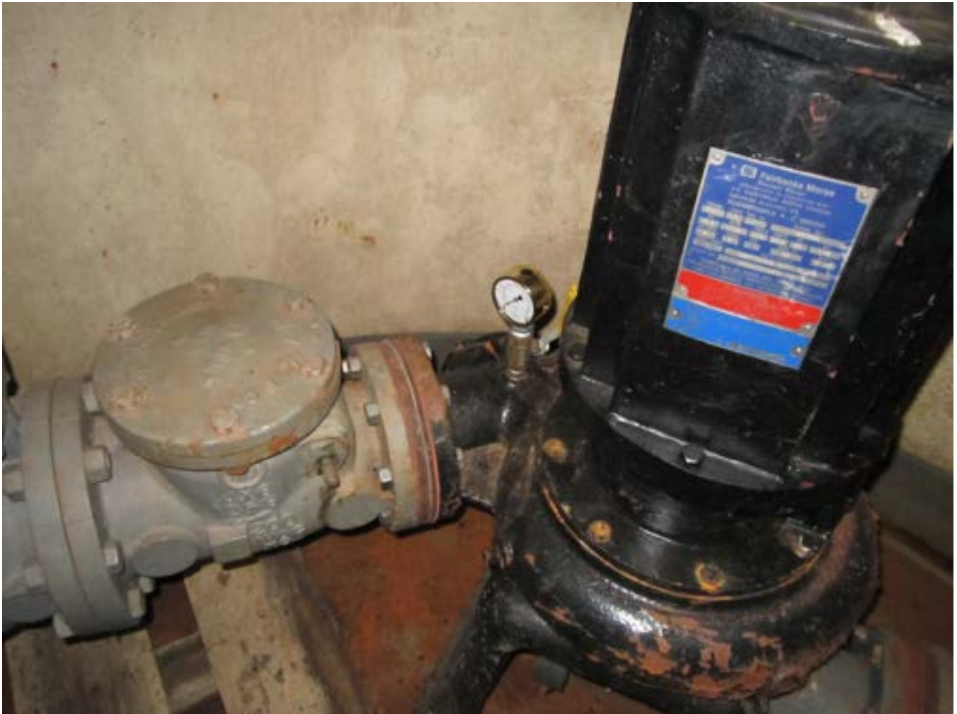
PHOTO 2: PUMP AND PRESSURE GAUGE
