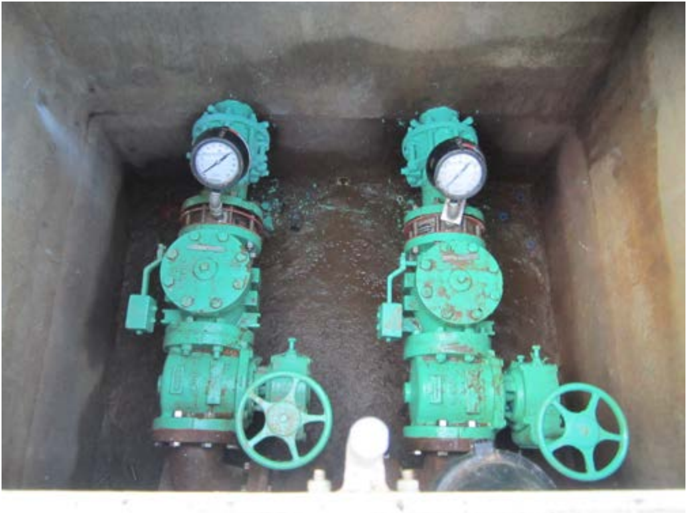
PHOTO 2: VALVE PIT PIPING AND PRESSURE GAUGES
