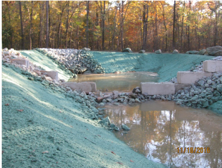
View of the first and second pools, facing upstream
