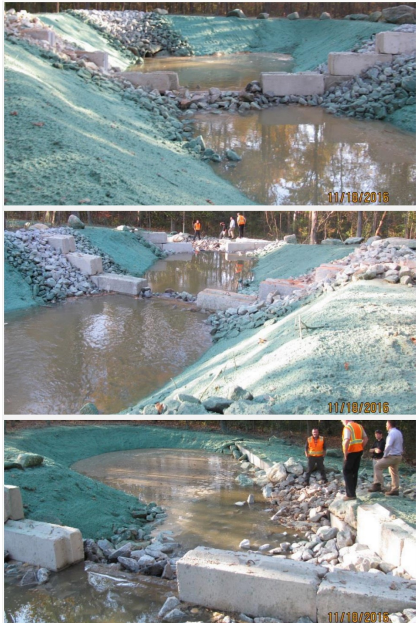
View during construction of the first and second pools, facing upstream (top); the first and second pools, facing downstream (middle); third pool, facing downstream (bottom).
