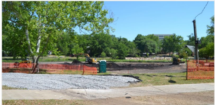
Silt fence installed at the start of construction to prevent sediment from entering Rocky Branch (upper two photos) and the construction entrance (bottom photo) located on Greene Street to prevent sediment leaving the site on truck tires and other equipment.
