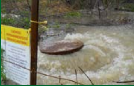
An extreme case of a wet-weather related SSO on the Columbia collection system
