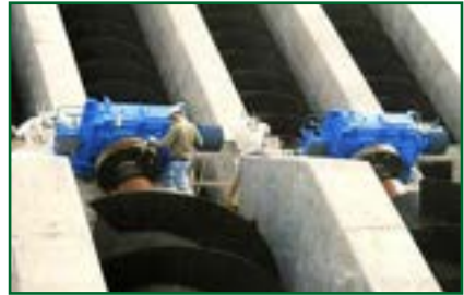
Technician installing screw pumps in the new headworks facility at Metro WWTP
