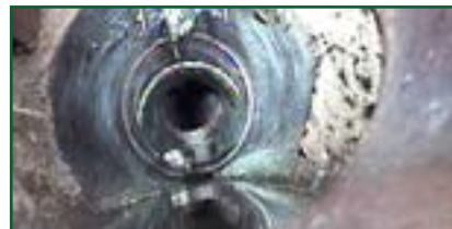
Section of missing pipe that has broken away, exposing the surrounding soil
