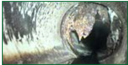
Plant roots entering pipe
